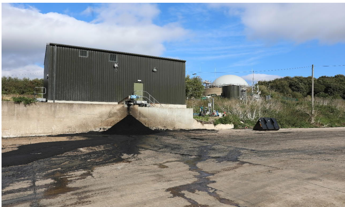
Figure J Sludge cake conveyors and pad
