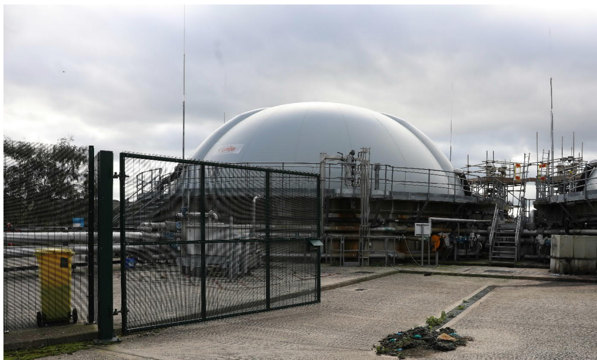
Figure H Anaerobic digesters
