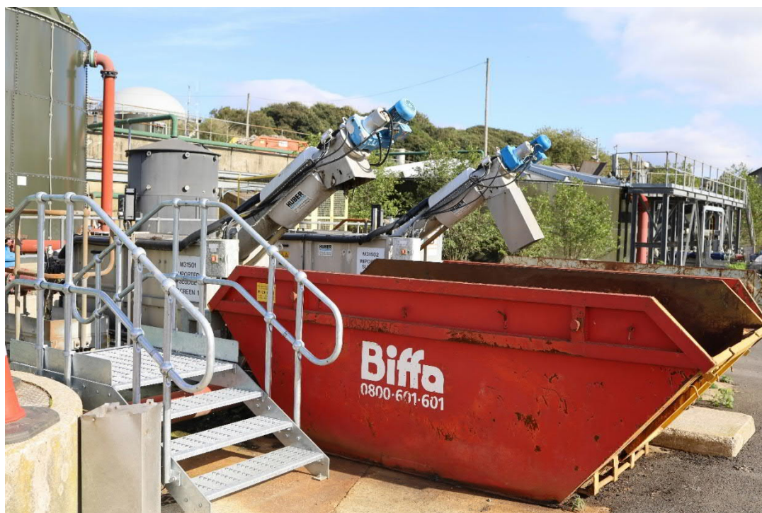
Figure D Sludge screens
