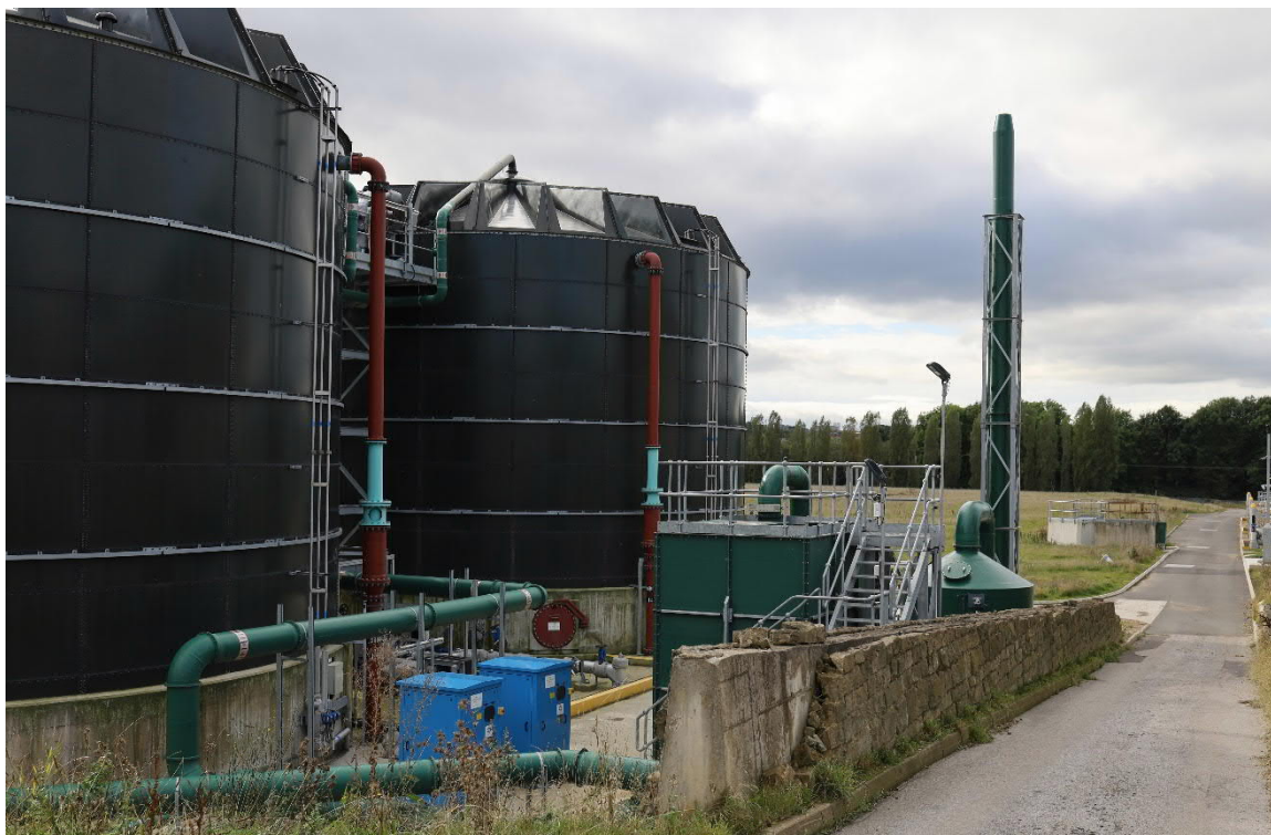
Figure E Thickener feed tanks and odour control unit
