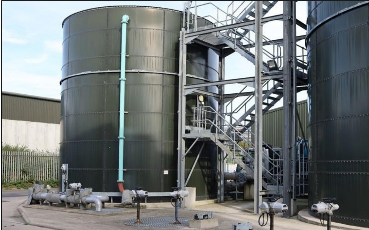
Figure 14. Liquor return tank.
