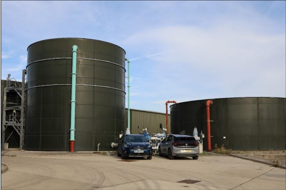
Figure 13. Dewatering feed tanks (2 no.).
