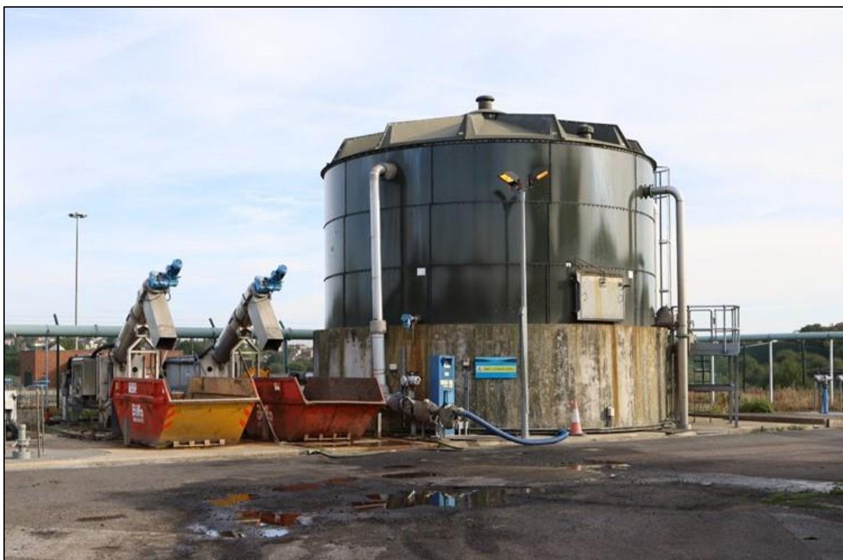
Figure 9. Sludge screen feed tank
