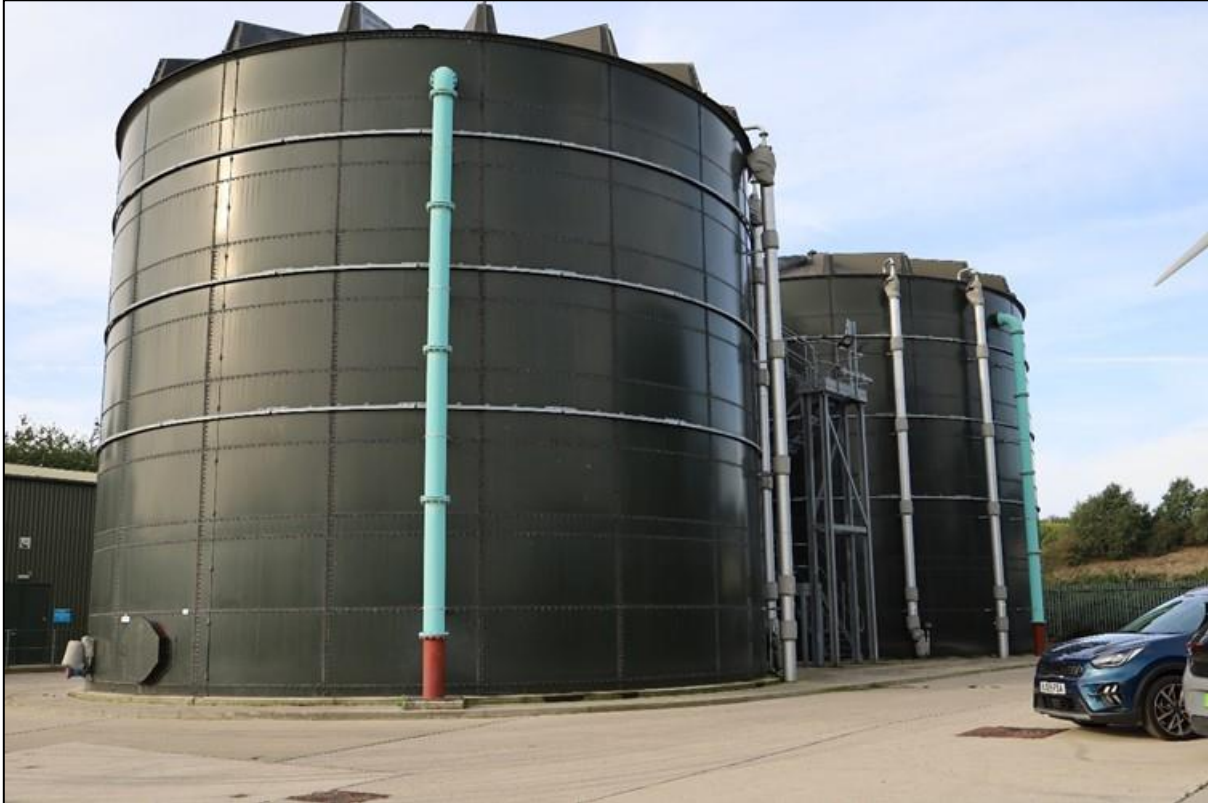
Figure 10. Drum thickener feed tanks (2 no.).
