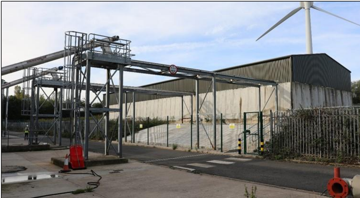
Figure 15. Digested sludge conveyer system.
