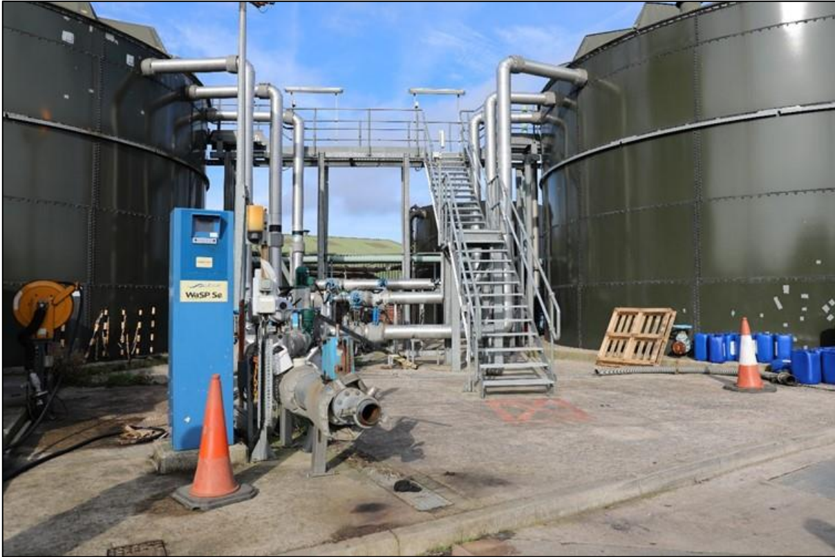
Figure 11. Digester feed tanks (2 no.).
