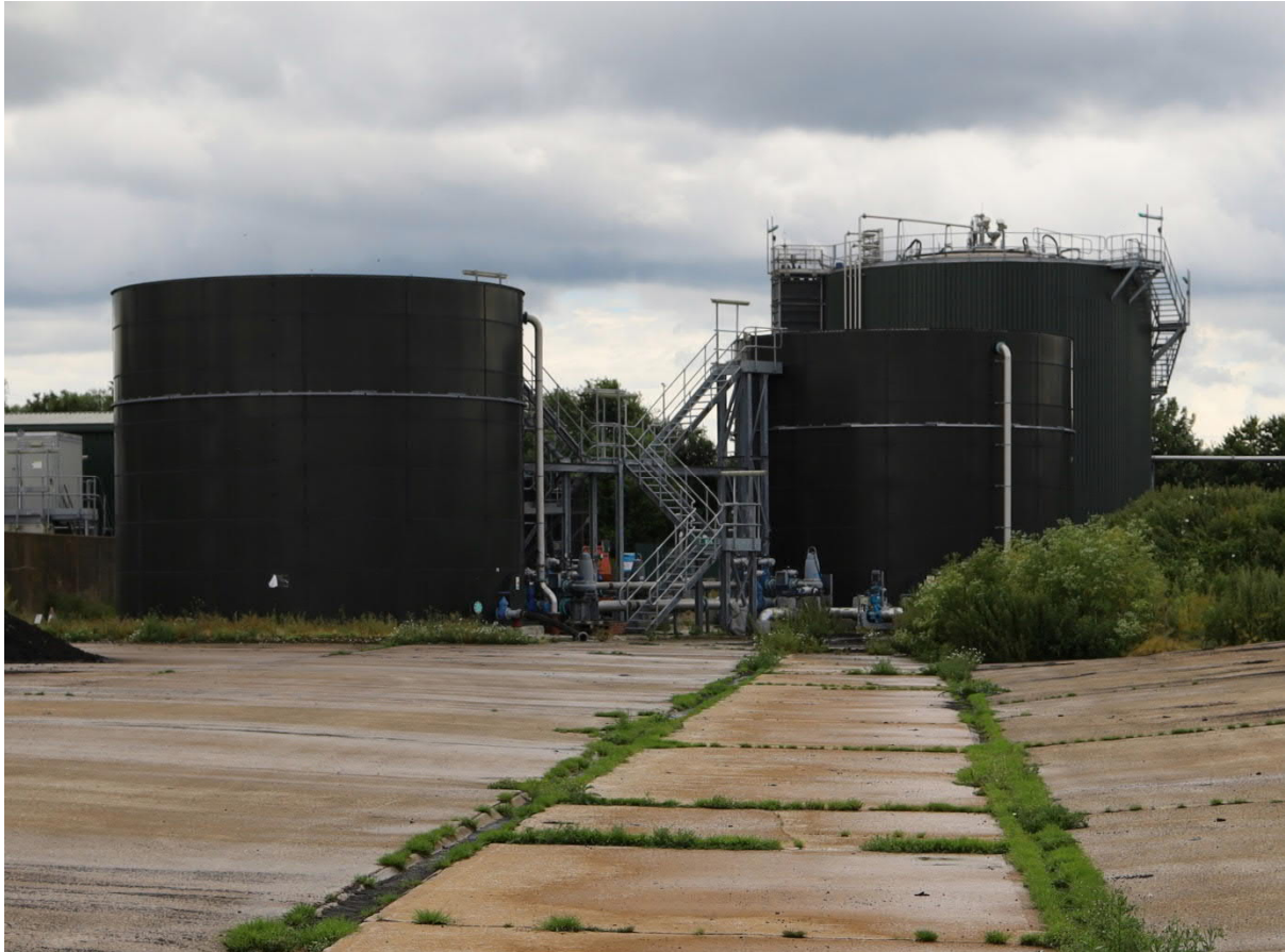
Figure 14. Dewatering tanks 2 and 3 (tanks in the foreground).
