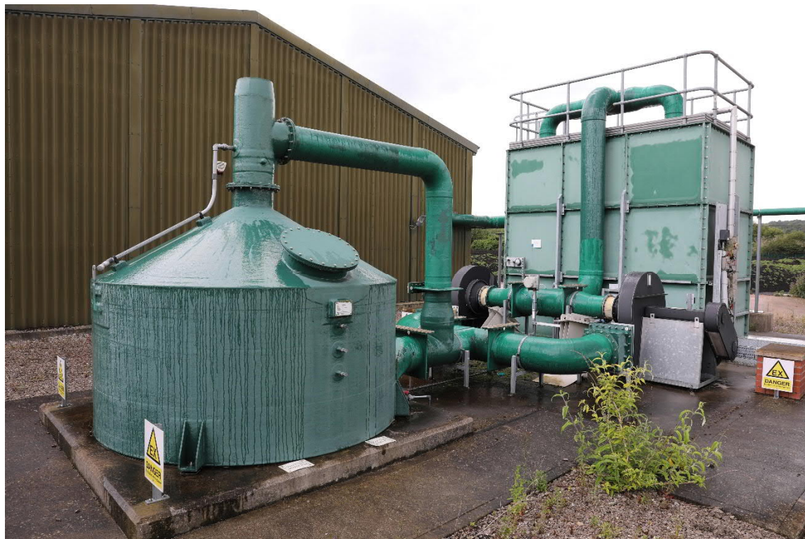
Figure F Odour control unit
