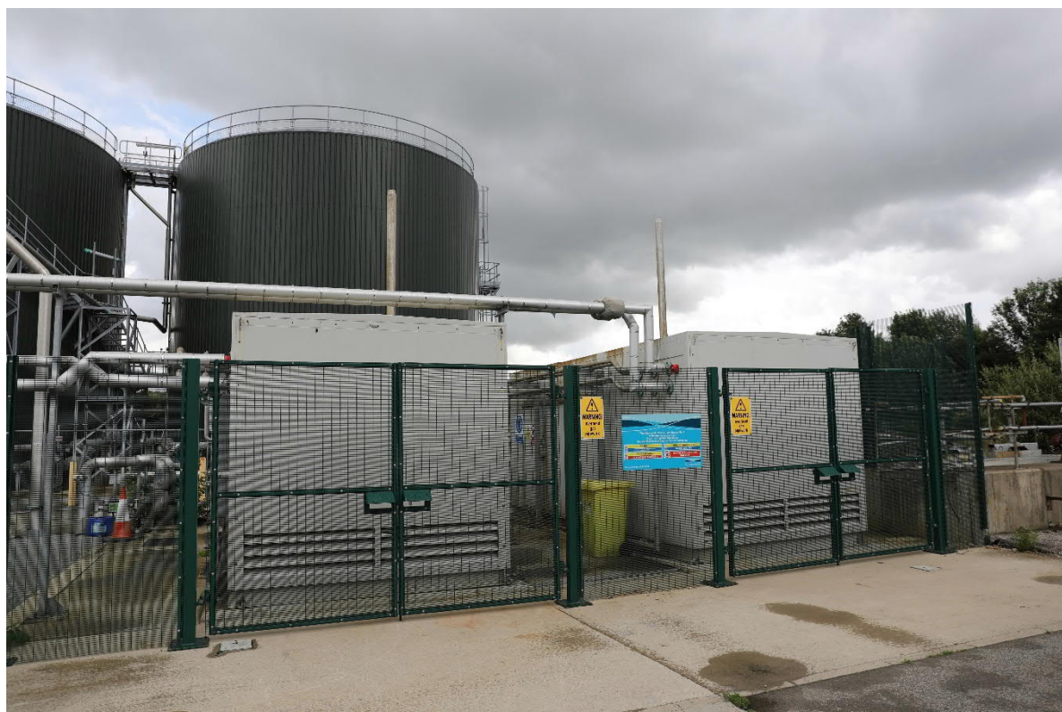
Figure G CHP units (with digesters behind)
