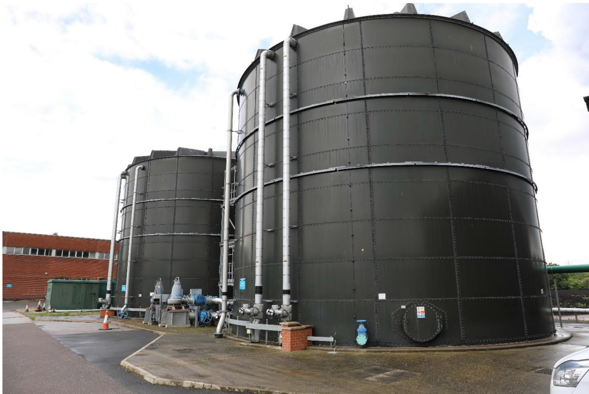
Figure 9. Thickener feed tanks (2 no.).
