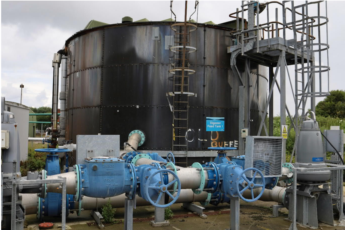
Figure 10. Digester feed tank 1.
