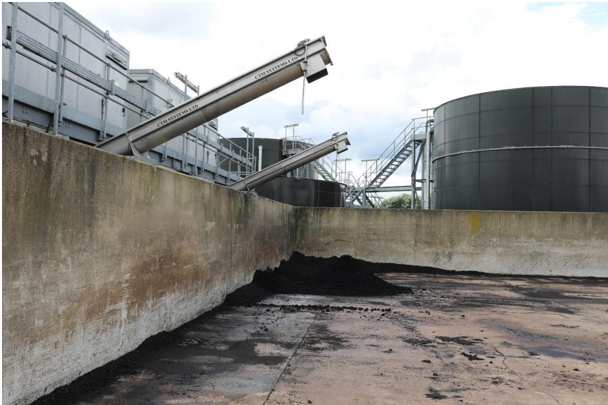
Figure 15. Sludge cake conveyors and pad.
