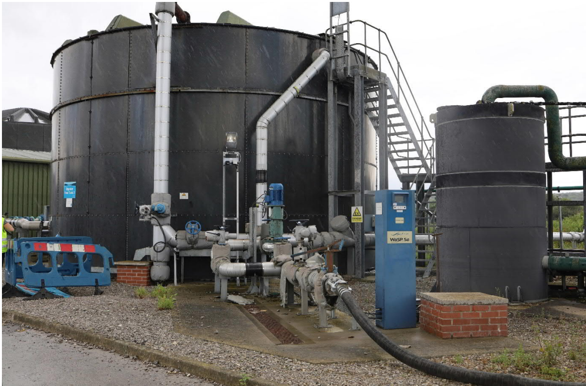
Figure 11. Digester feed tank 2.
