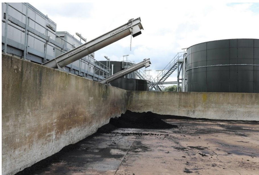
Figure 1 Sludge cake conveyors and pad
