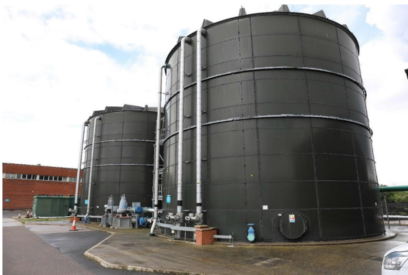
Figure D Thickener feed tanks
