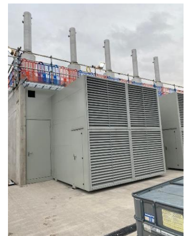
Air inlet unit
