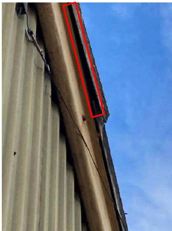
Plate 10. Gap beneath roof overlap on western gable end
