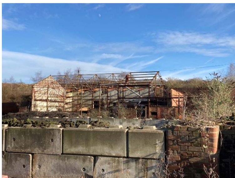
Plate 8. Example of a derelict building within the Site
