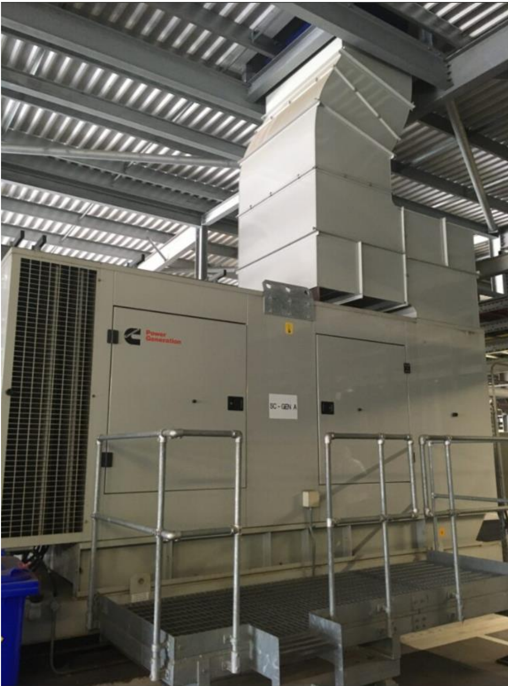
Figure 1: Crawley Unit 1 data centre diesel shell and core (landlord) standby generator
