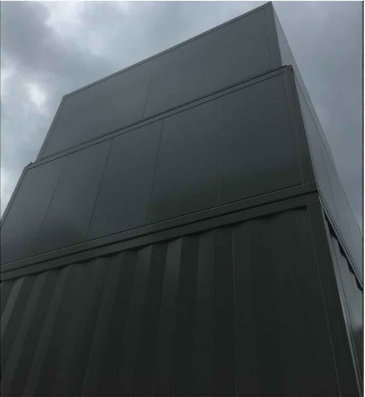
Figure 12: Crawley Unit 2 diesel Standby Generator stack height
