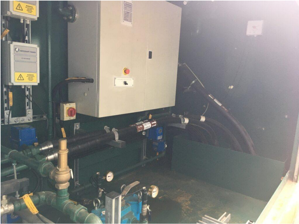
Figure 6: Crawley Unit 1 aboveground tank fill points and alarms within fill point cabinet
