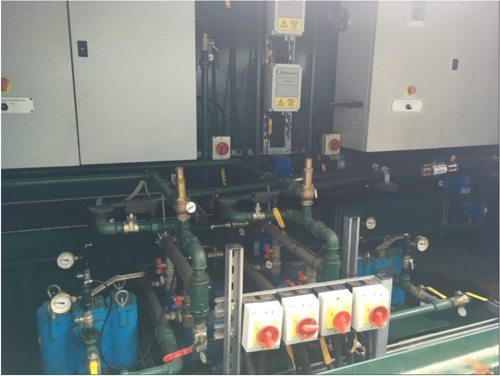
Figure 5: Crawley Unit 1 aboveground tank fill points and alarms within fill point cabinet
