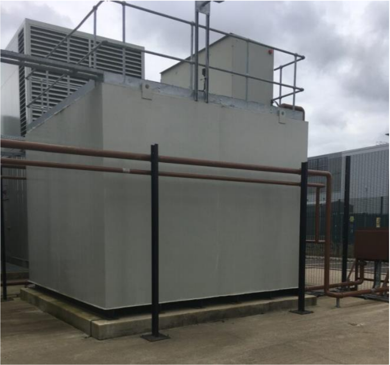
Figure 11: Crawley Unit 2 diesel Standby Generator
