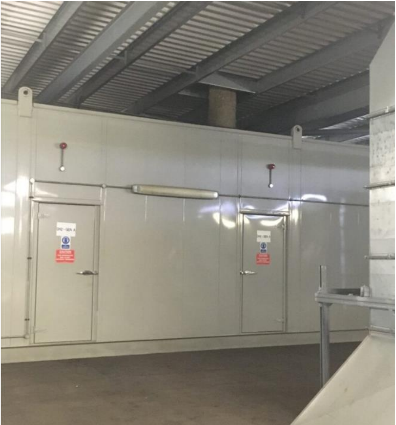
Figure 10: Crawley Unit 1 diesel Data Hall Standby Generator
