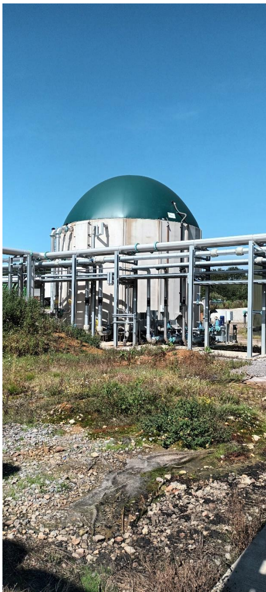
Photograph 14: New raw waste buffer tank with aboveground pipework. Secondary containment to be completed.
