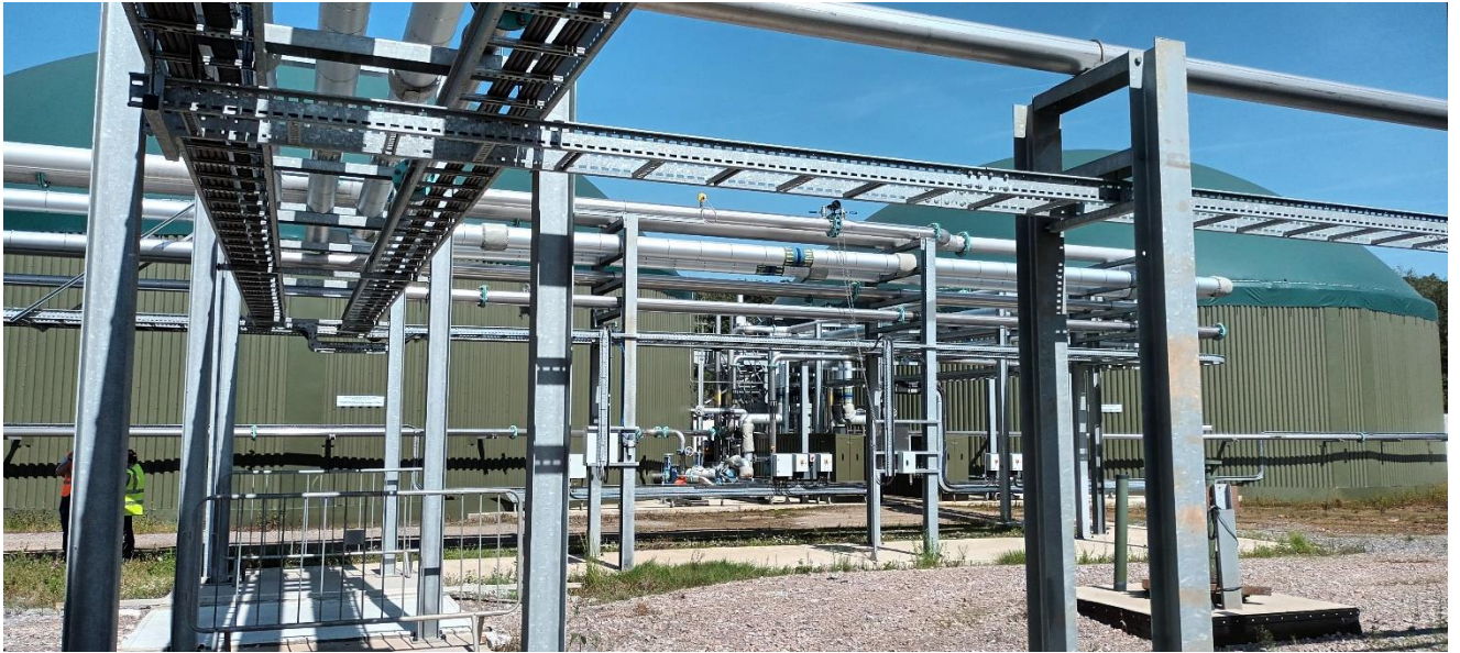
Photograph 15: D2 and D3 with supported aboveground pipework
