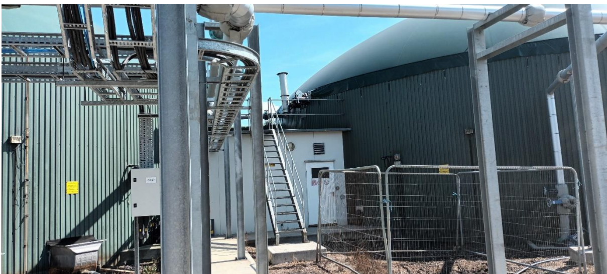
Photograph 13: Above ground pipework associated with Digester 1 and Post Digester
