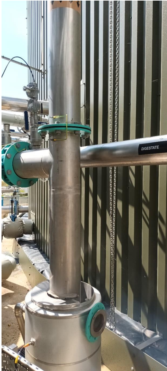
Photograph 19: Foam pot on new digester
