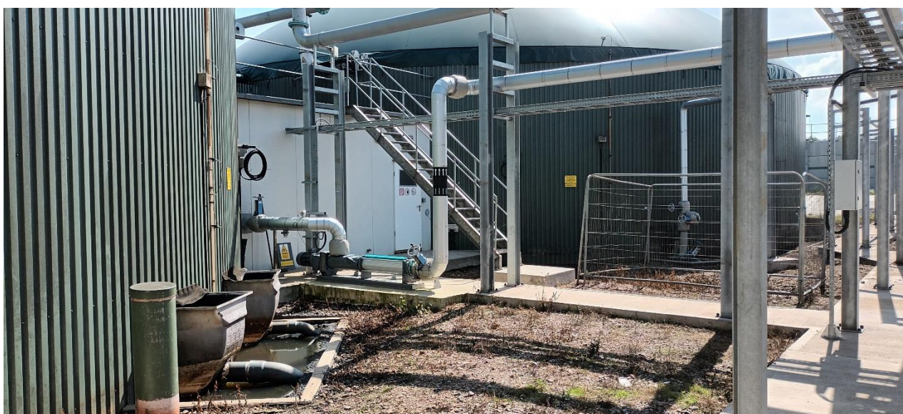
Photograph 10: Post digester & digester 1 with control room between. Leak detection pots
