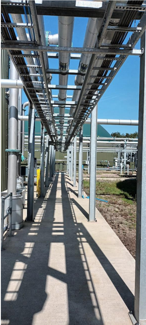
Photograph 12: Above ground pipework associated with new pasteuriser and 2 new primary digesters (D2 & D3)
