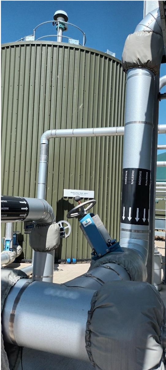
Photograph 11: New single pasteuriser tank
