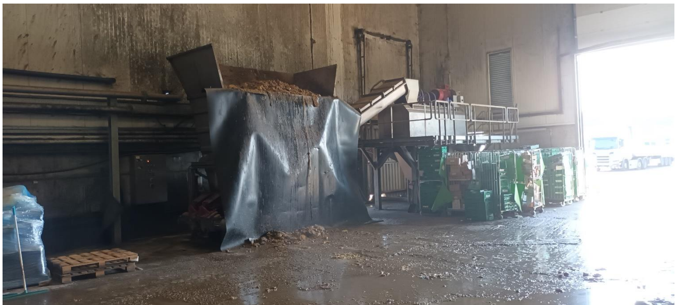
Photograph 4: Solid food waste hopper and depackaging plant in waste reception building
