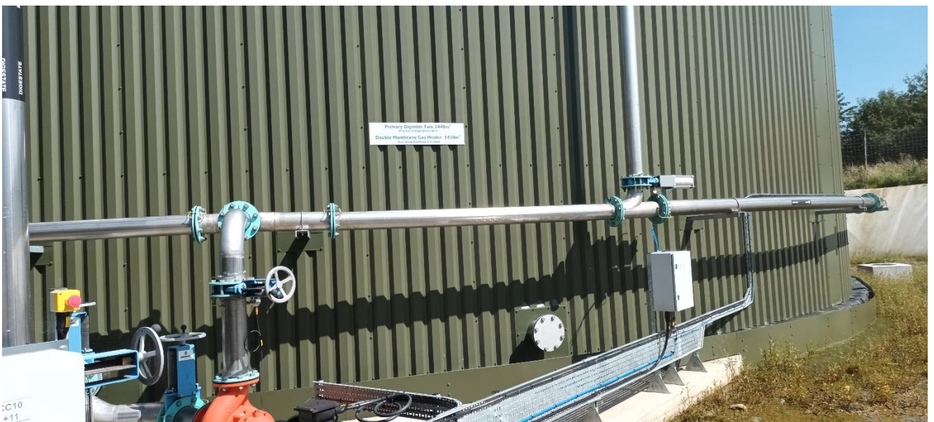
Photograph 18: D2 with new secondary containment bund beyond
