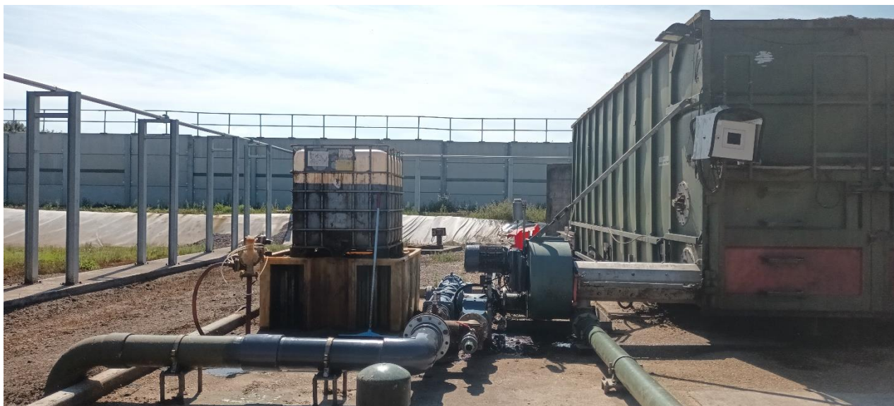
Photograph 9: Crop feeder with northern silage clamp wall and secondary containment liner for existing plant in foreground
