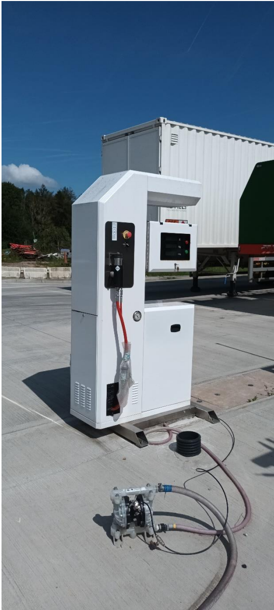
Photograph 21: Refuelling pump (not in use)
