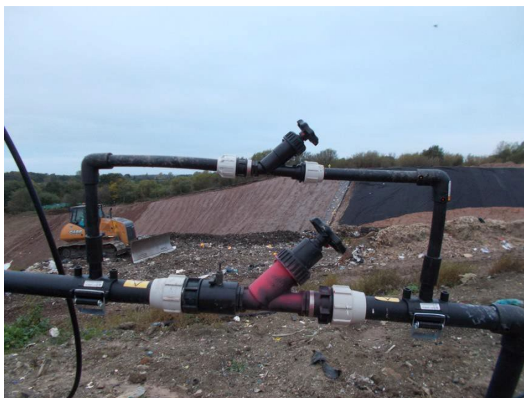
Plate 2: Bleed over gas control system as installed onto a leachate chamber
