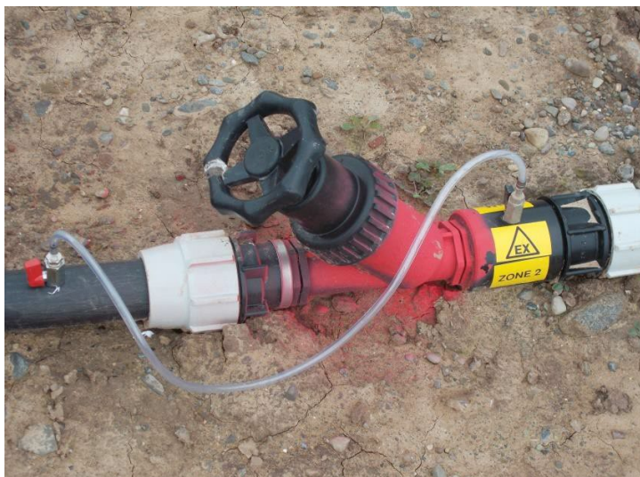
Plate 1: Bleed over gas control system installed on an odour control gas extraction point.
