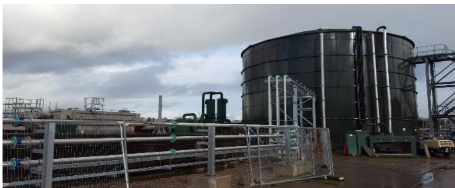
Photo 7 - EEH feed tank and OCU
