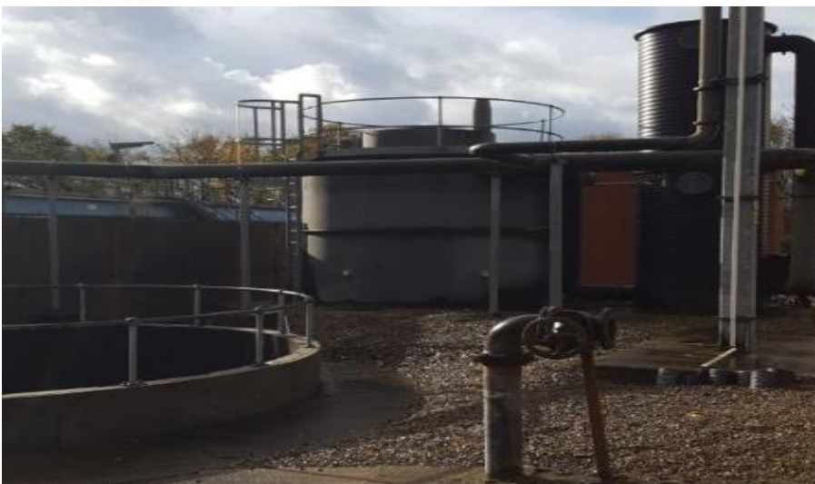
Photo 5 – OCU connected to the unthickened sludge tank
