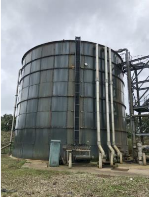
Photo 4 – Unthickened sludge storage tank
