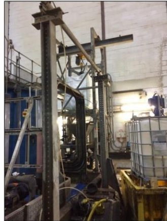
Figure 12: Polyelectrolyte hopper, dryer building
