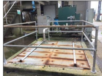
Figure 8: Cess inlet wet well
