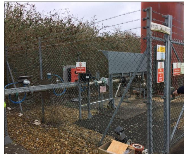
Figure 18: Flare stack compound
