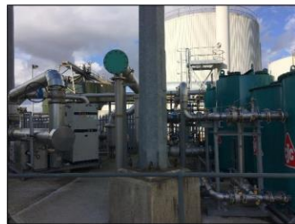
Figure 17: New CHP plant
