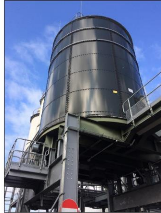
Figure 13: Post digestion sludge cake storage silo
