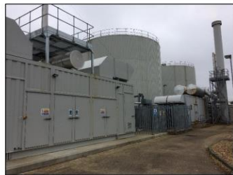
Figure 16: Existing CHP plant
