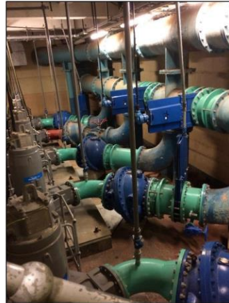
Figure 2: PS3 inlet works dry well
