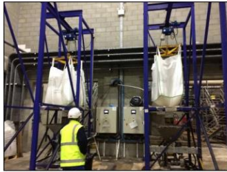
Figure 11: Polyelectrolyte hoppers, located next to boiler room.
