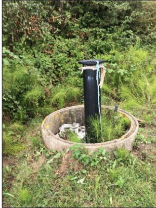
Figure 23: Gas sampling point.
