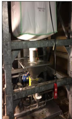
Figure 13: Polyelectrolyte dispenser 3, centrifuge building.
