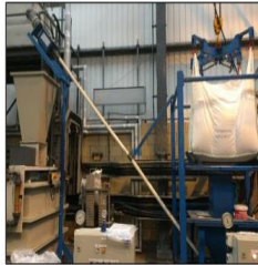
Figure 11: Polyelectrolyte dispenser 1, chemical building.
