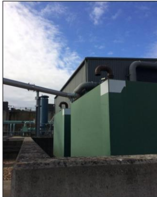
Figure 22: Diesel tanks, secondary treatment.
