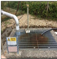
Figure 18: Condensate trap, flare stack.
