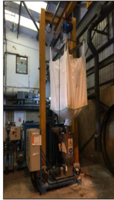
Figure 12: Polyelectrolyte dispenser 2, next to boiler house.
