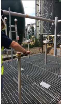
Figure 17: Condensate trap, digesters.
