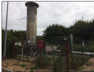
Figure 16: Flare stack compound.
