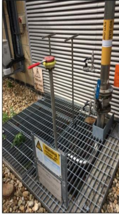
Figure 19: Condensate trap, boiler house.
