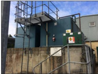
Figure 21: Diesel tanks, primary treatment.
