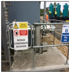
Figure 20: Gas condensate receiver.
