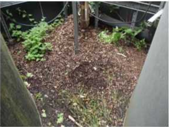
Photograph 8: Significant vegetation in and around tank bunds.
