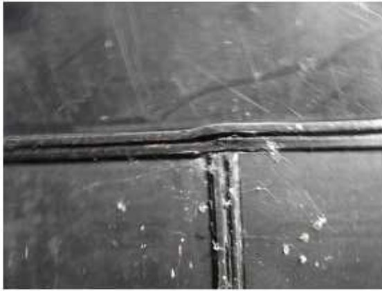
Photograph 13: The internal tank bund shell is in good condition with all welds well made.
