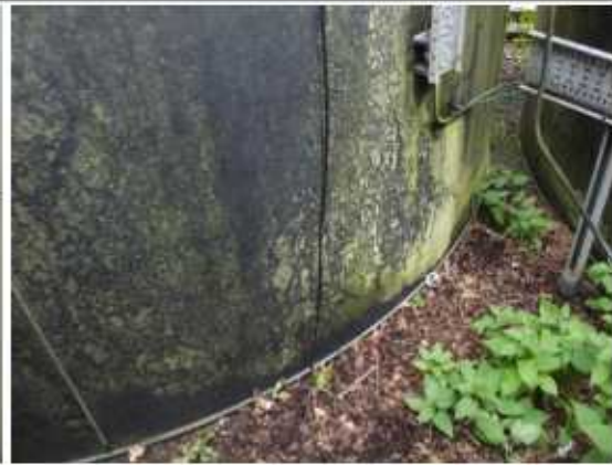
Photograph 4: Tank bund is installed directly on top of the foundation.
