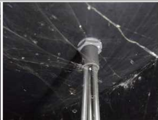
Photograph 16: Bund lid penetration – potential source of rainwater ingress.
