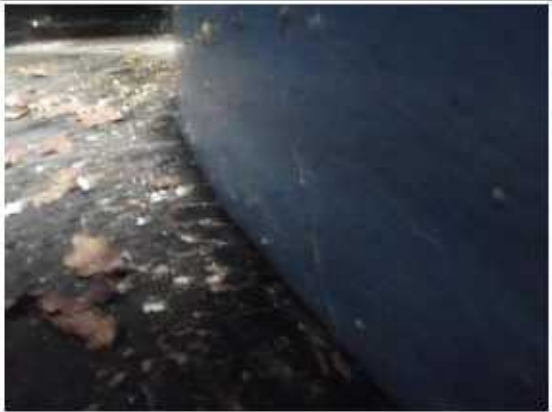
Photograph 7: The tank is installed directly above the plastic bund floor, above a concrete base.
