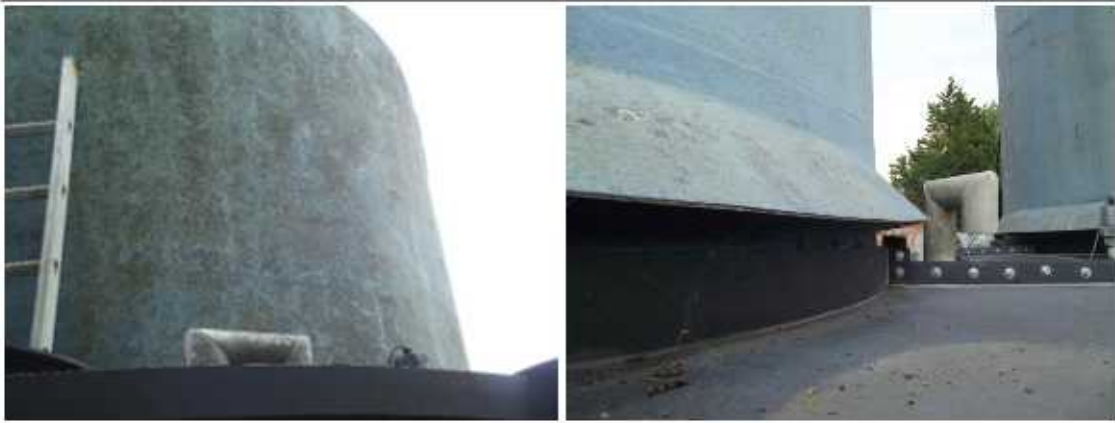
Photograph 9: The tank shell above the bund is in good condition – note fungal growth. Photograph 10; Fibre glass rain-deflector skirt is in good condition – note fungal growth.
