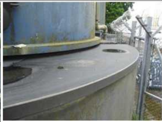
Photograph 9; Mild-steel rain-deflector skirt above bund lid.
