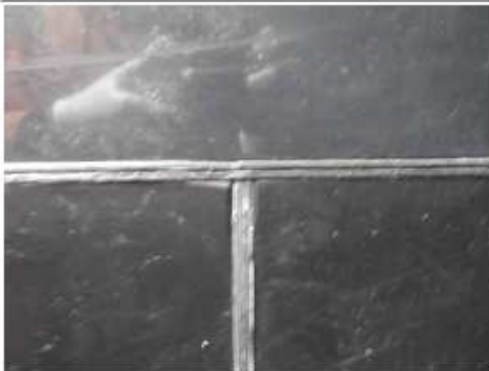
Photograph 13: The internal tank bund shell is in good condition with all welds well made.
