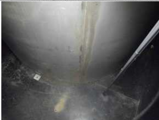
Photograph 10: The external shell below the bund is in good condition and unpainted.
