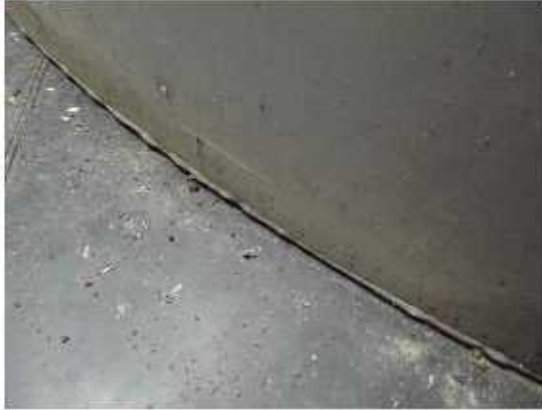
Photograph 6: The tank is installed directly above the plastic bund floor, above a concrete base.
