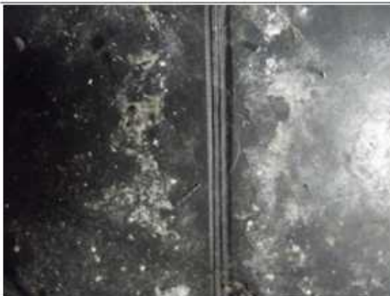
Photograph 14: The tank bund bottom is clean and dry. Welds all well made.
