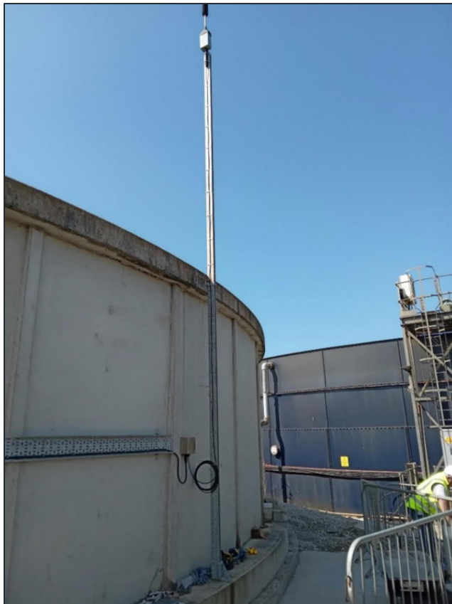
Figure 5-6 – Photo of Noise Monitoring Equipment
