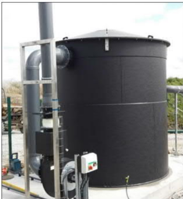
Figure 4-22 – Photograph of OCU at Contingency Lagoon
