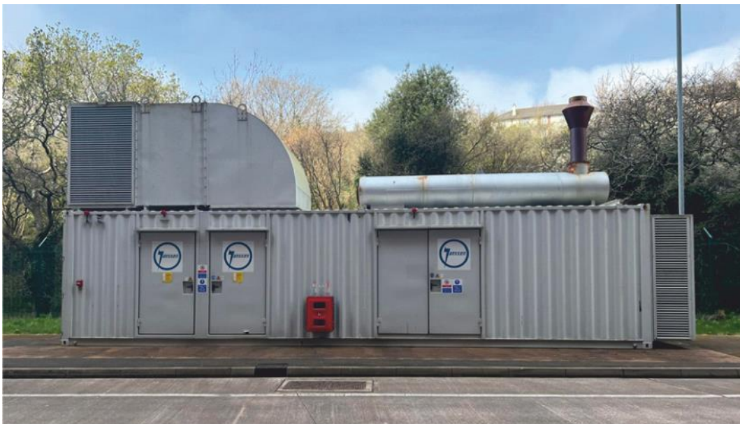
Graphic 3.12: A typical emergency diesel generator
