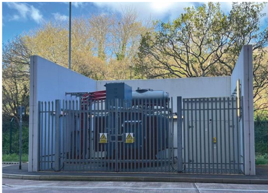
Graphic 3.11: A typical mains transformer compound
