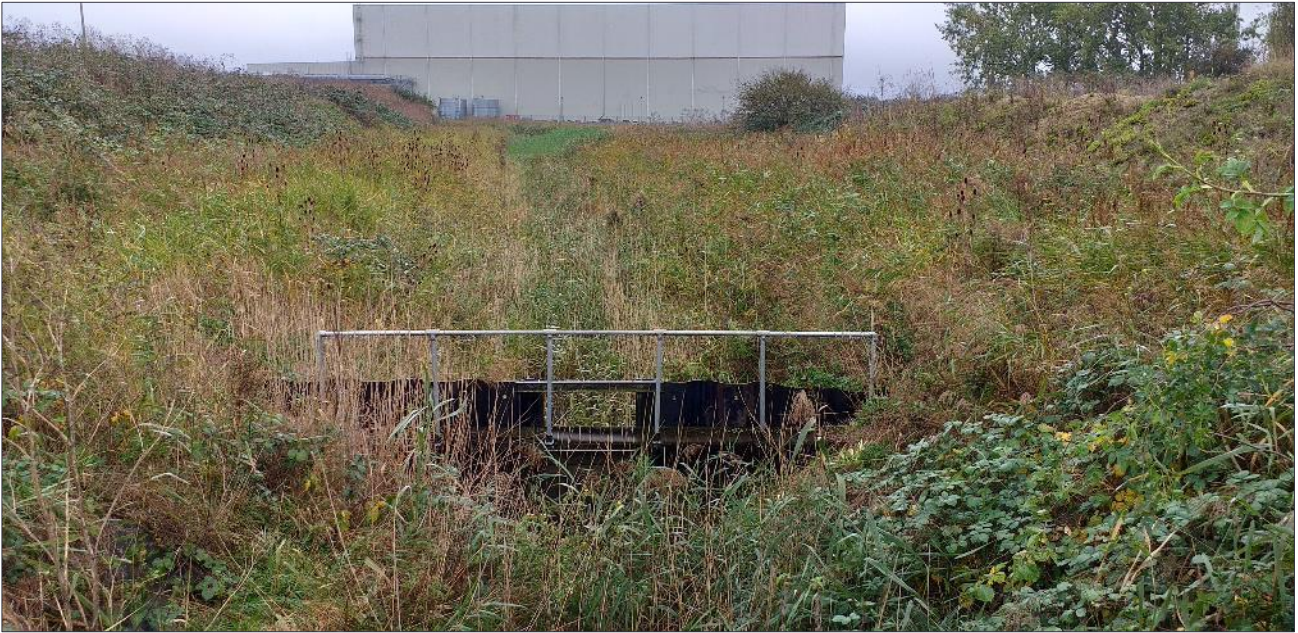
Looking south-east along the drainage channel separating Areas A and B of the site.
