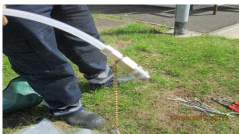
Air release valve disconnected
