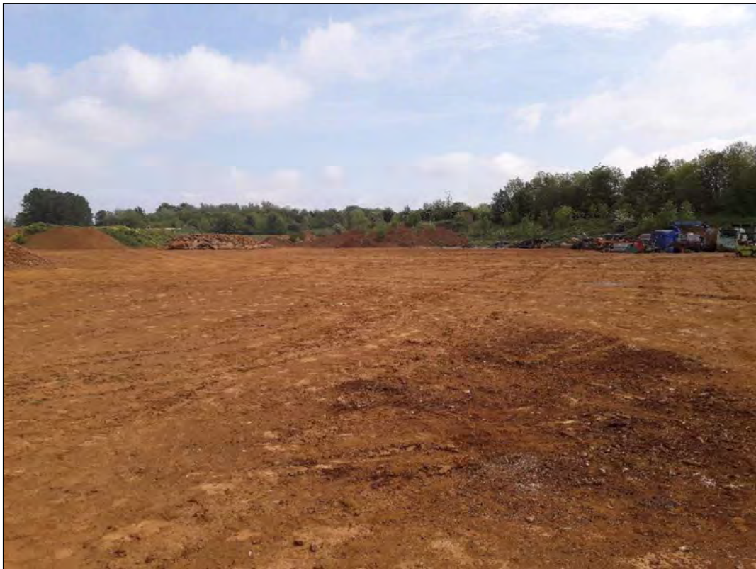
View across site from southern site boundary with parked trucks in right of view (view to northeast)
