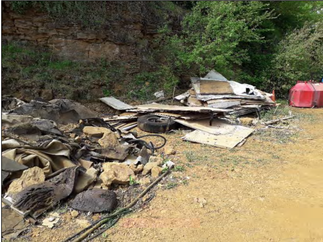
Segregated waste in southwest of site with fuel tank in right of view (view to south)
