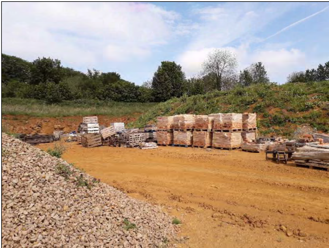
Packed pallets of screened aggregate in northwest of site (view to northwest)
