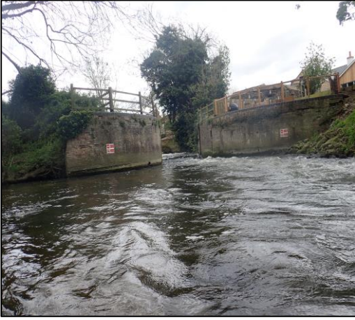
Photograph seven: View looking upstream towards Turf Lock (from within the river channel in a boat), April 2024
