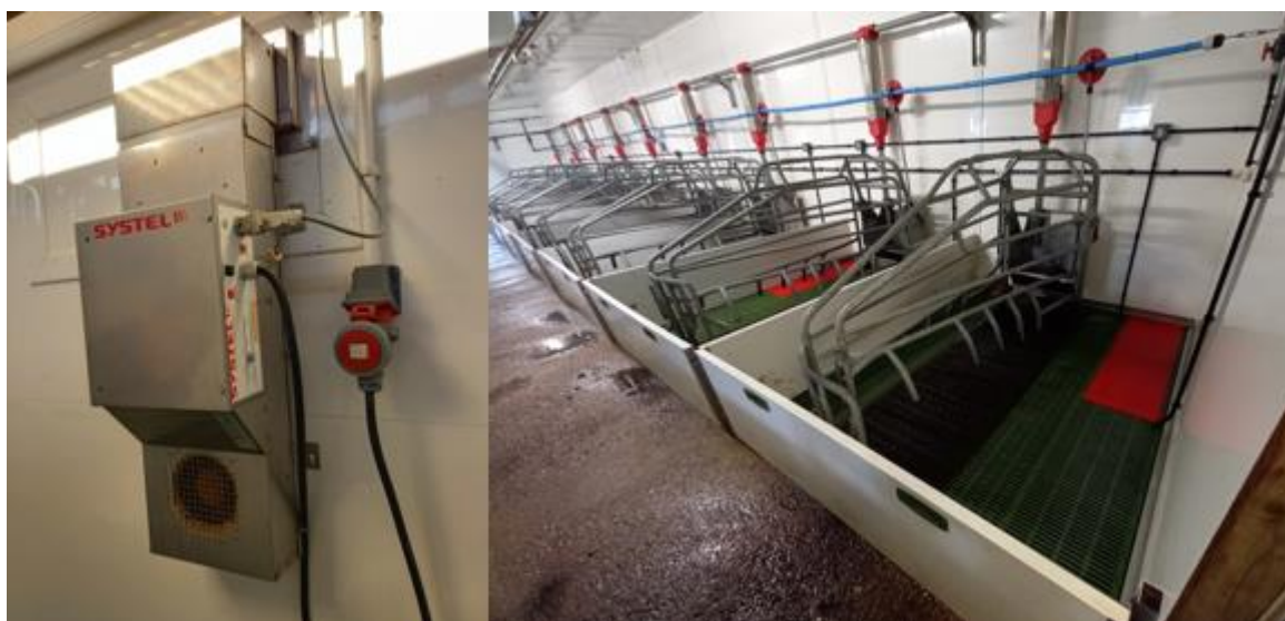
Figure 8 showing a mobile 10kW fan heater left & the red 120W heating pads in the farrowing rooms
