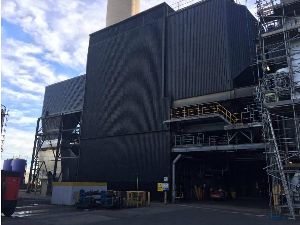
Figure 3: Electrostatic Precipitators (Unit 1 ESP from Boiler House - right, to ID Fan Inlet - left)
