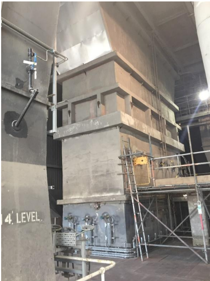
Figure 8: Boiler House at 114' Level showing Economiser to Air Heater Ductwork (High Dust SCR Location)
