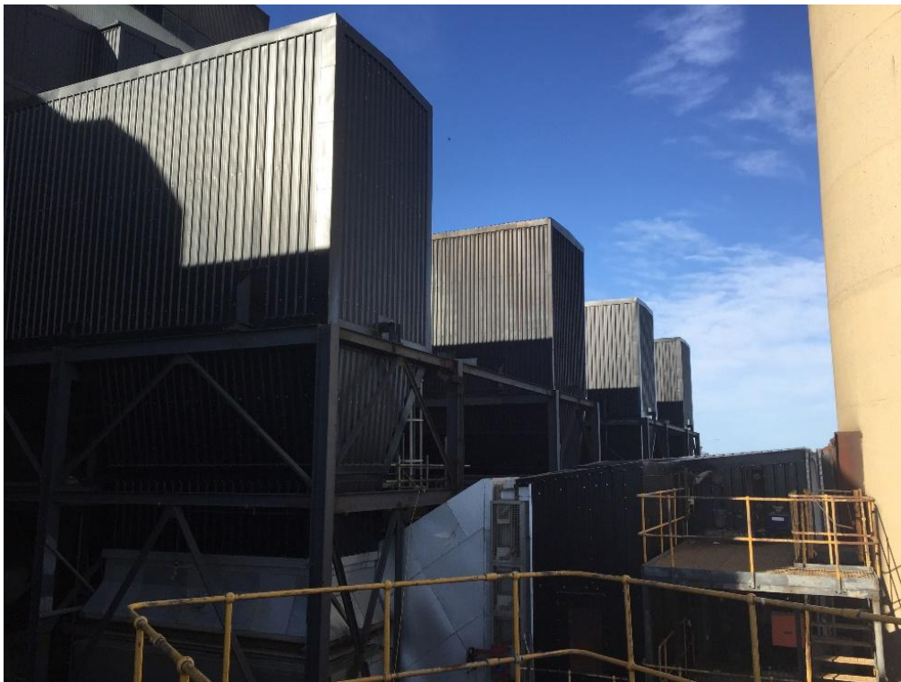
Figure 2: Electrostatic Precipitators (Showing Close Proximity of Unit 1 & 2 ESP Outlets and ID Fan Ductwork to Stack Inlet)
