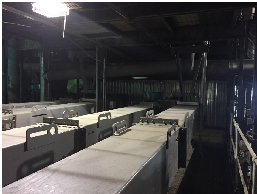
Figure 6: Potential Boiler Sidewall Reagent Injection Locations Demonstrating Restricted Access Due to Existing Sootblowers (Unit 1 Final Reheat Level)
