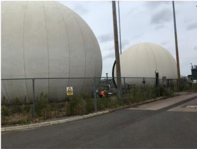
Photo showing the Biogas Storage holders, with lightning protection wires. The Biogas Storage holders receive biogas from the PDTs and the biogas is then combusted on site.
