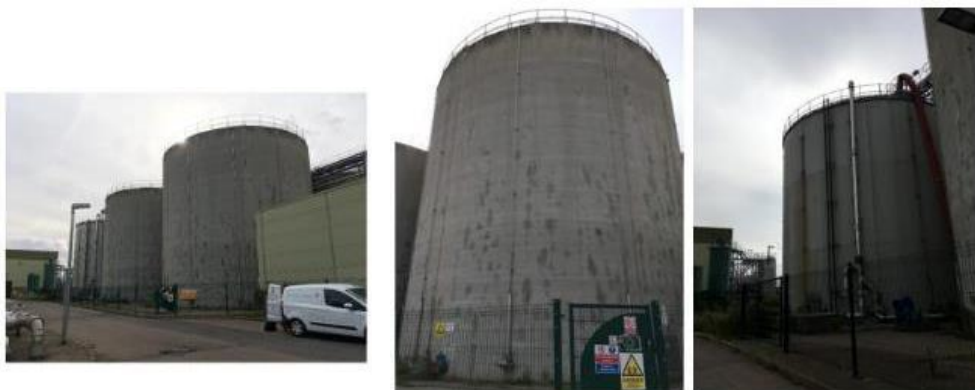
Photos showing the general view of the Primary Digester Tanks with fixed roofs surrounded by hardstanding. There are nine tanks in total, with eight Primary Digester Tanks of concrete construction and one Primary Digester Tank of steel construction.
