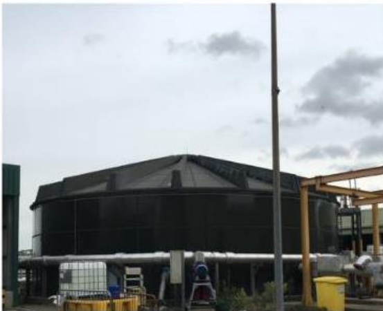
Photo showing the Sludge Blending Tank. The Sludge Blending Tank receives thickened sludge, thickened SAS and screened imported sludge. Blended sludge is then pumped to the Primary Digester Tanks (PDTs).
