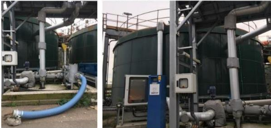
(Left) Photo showing the Sludge Import Point on hardstanding with bunding. (Right) Photo showing the Sludge Import Tank in the background with the import logger in the foreground.
