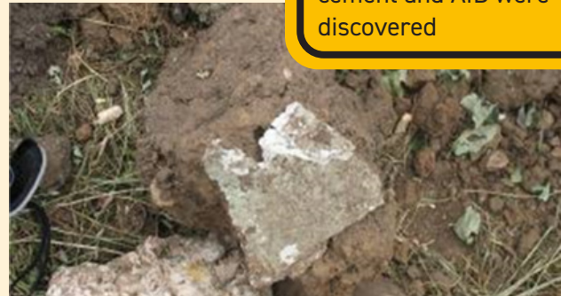
Asbestos finds | Ramboll
