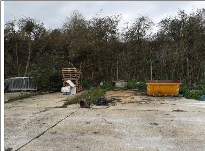
Storage area, some staining on hardstanding
