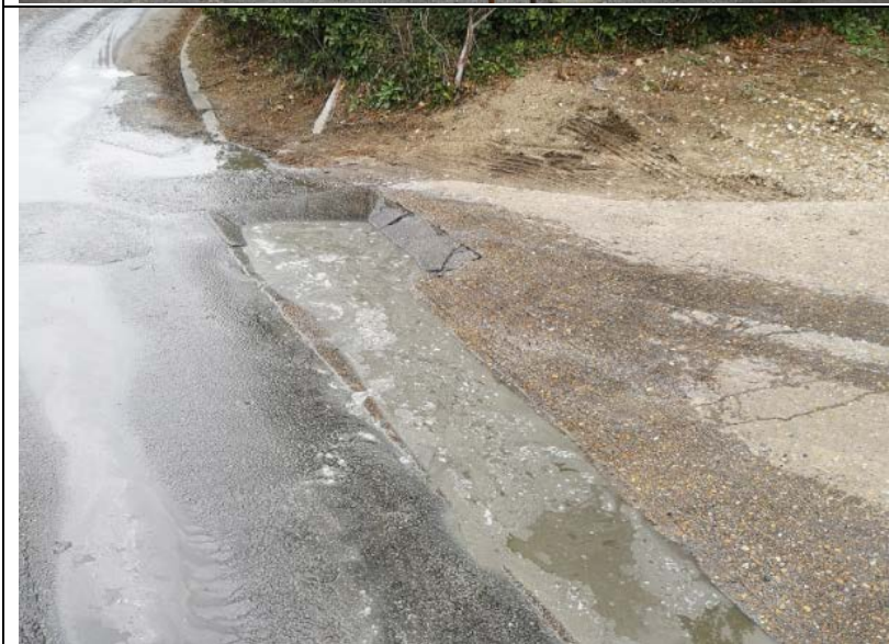
Blocked drains noted on site
