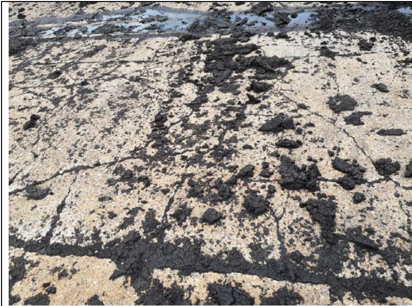
Cracked hardstanding in cake bays
