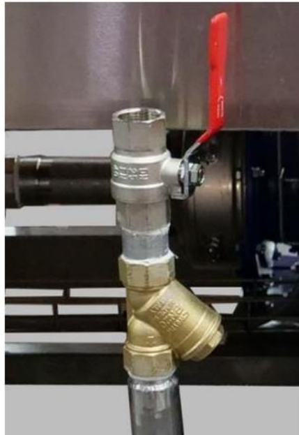
Figure 12 – Water Supply IN Valve
