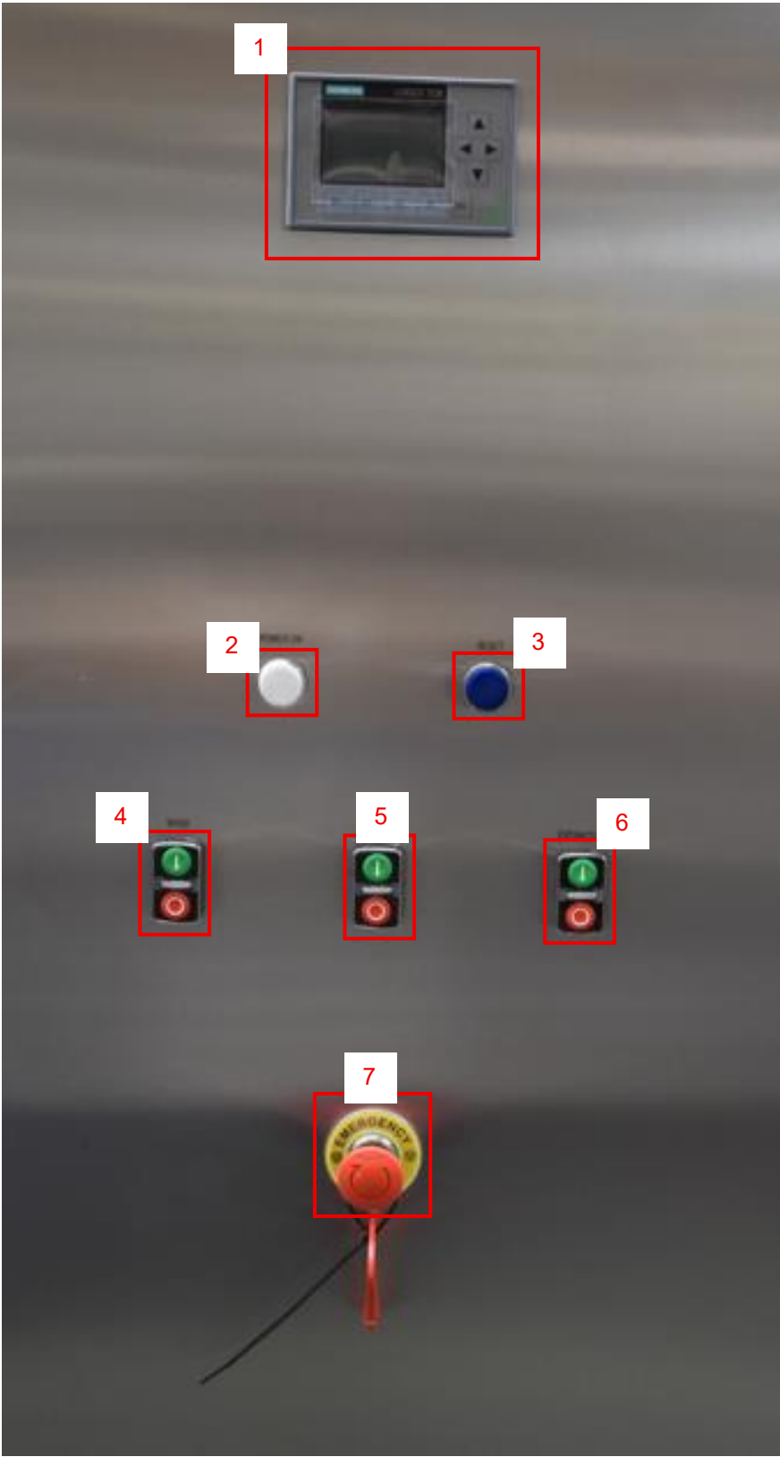
Figure 19 – Exterior of Control Panel
