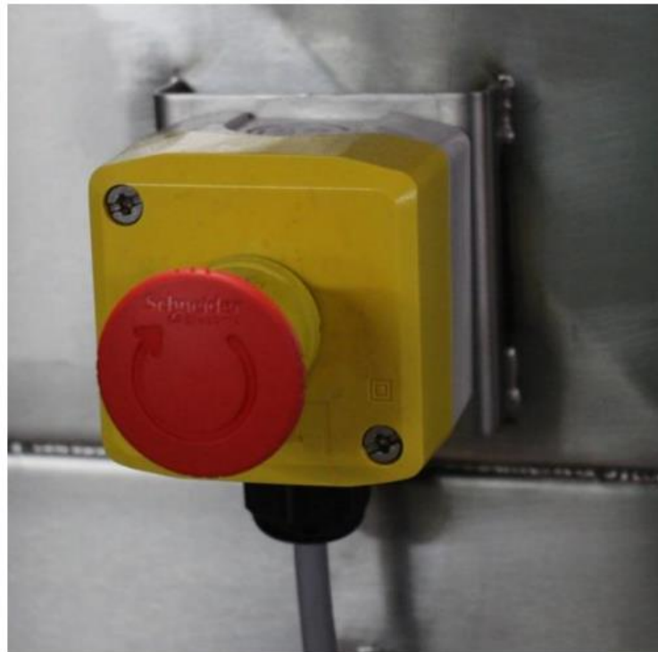
Figure 13 – Emergency Stop Pushbutton
