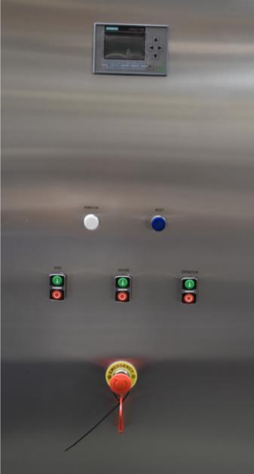
Figure 4 – Exterior of Control Panel
