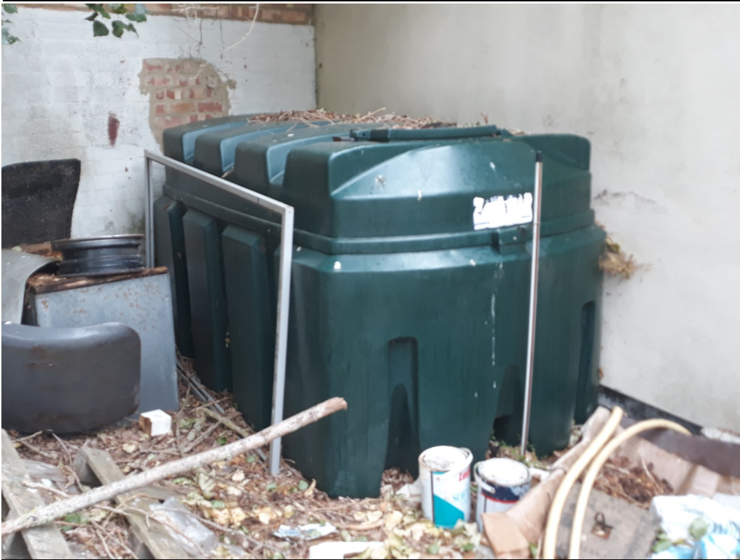
Photo 3—2500l kerosene AST for heating system.
