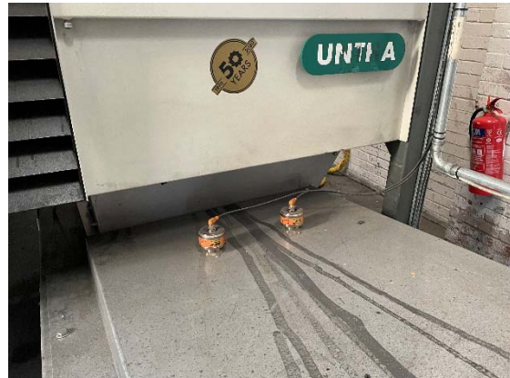
Photo 8: Fire sensors to allow 2 sec bursts of water to be deployed until fire extinguished
