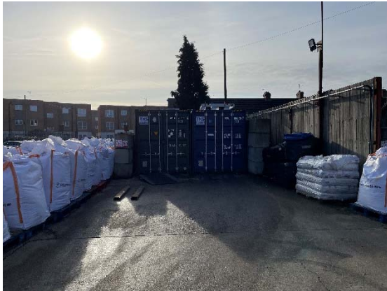
Photo 1: Temperature controlled shipping containers for battery storage and FIBC lithium flake storage
