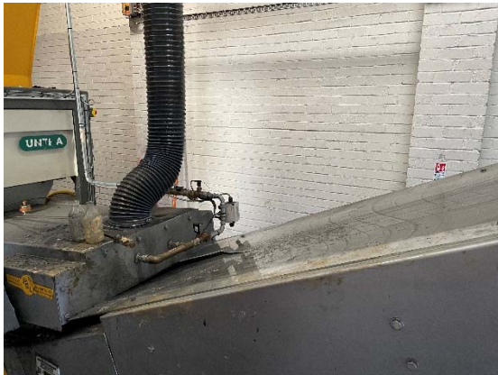
Photo 7: Shredded material passes along covered conveyor
