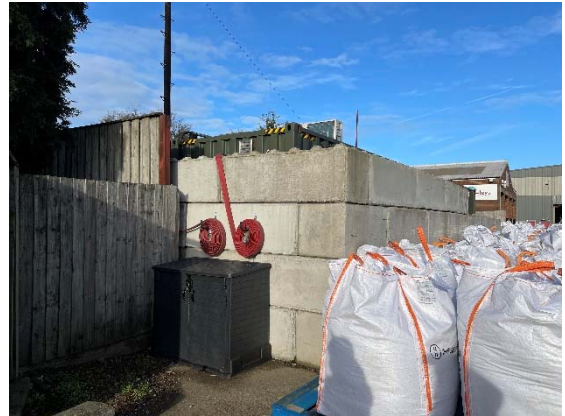
Photo 2: Fire break walls around temperature-controlled shipping containers and hose connections to flood containers with water in event of thermal runaway
