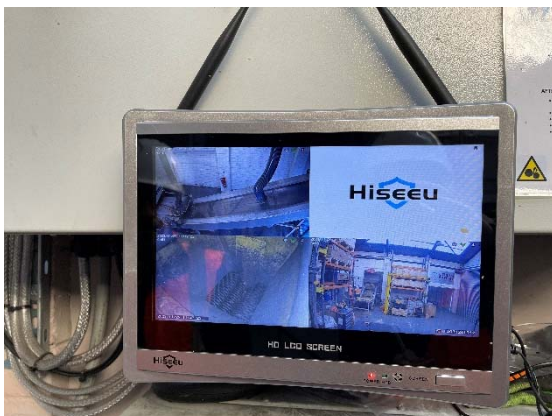
Photo 5: Process monitored remotely via cameras
