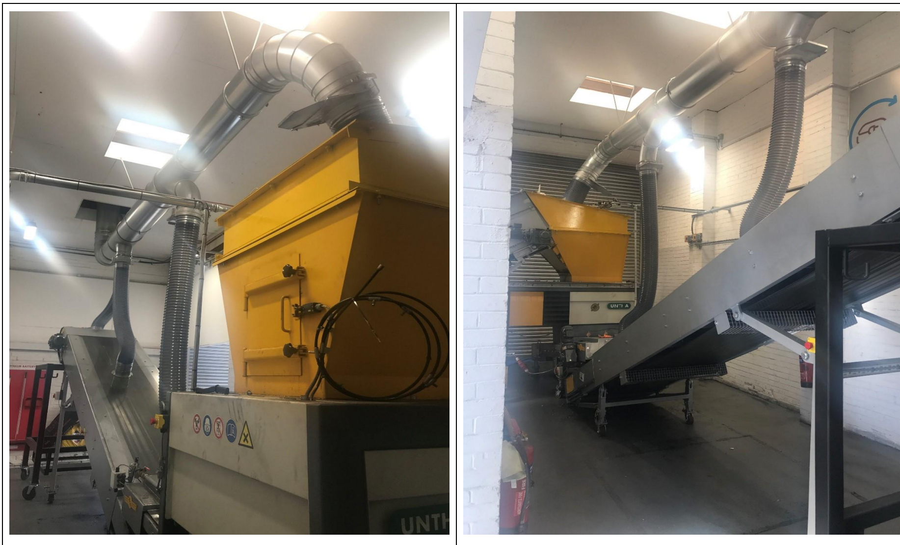
Photograph 1: Shredder hopper, enclosed product (belt) conveyor and LEV ducting.
