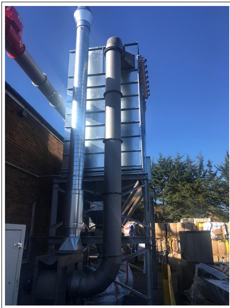
Photograph 3: Dust Extraction Unit including spark detection system (red colour, top left) on inlet piping.
