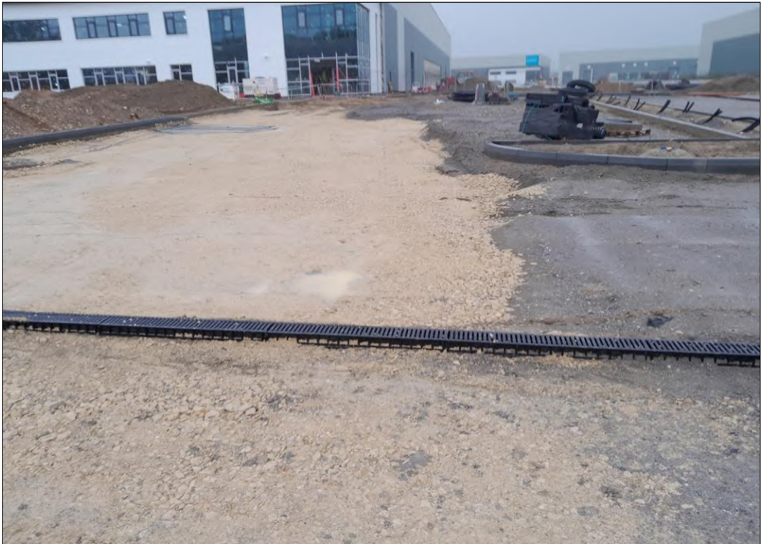
Photo 1 – Eastern zone of removed IBAA, fully replaced with NFS looking to the west.
