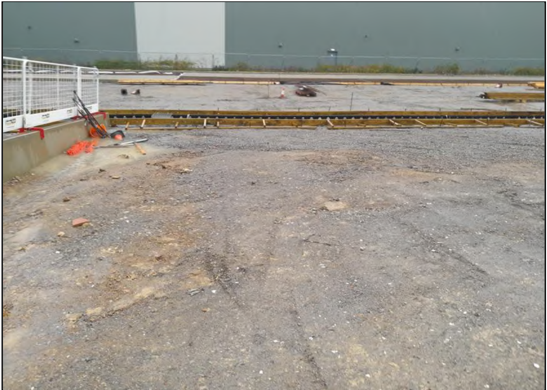
Photo 5 – Extent of IBAA from the division along the loading bay division.
