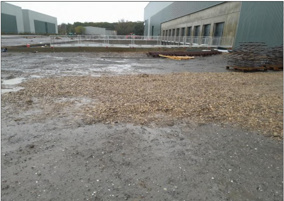
Photo 6 – IBAA present across the southwestern zone, gravel present from vehicle entry to warehouse construction.
