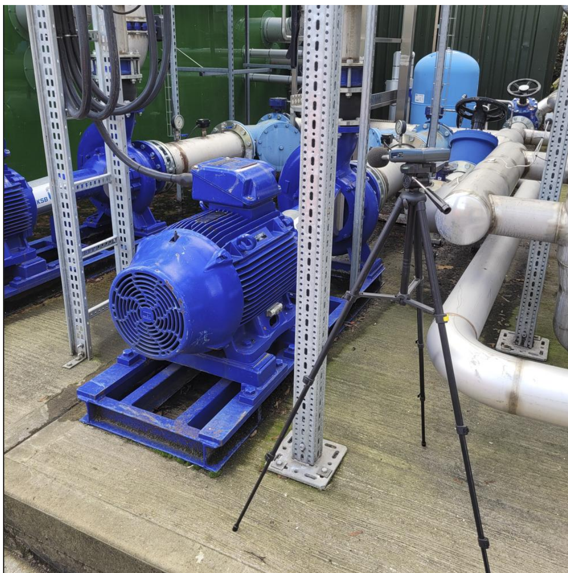
Figure D10: Refrigeration Pumps
