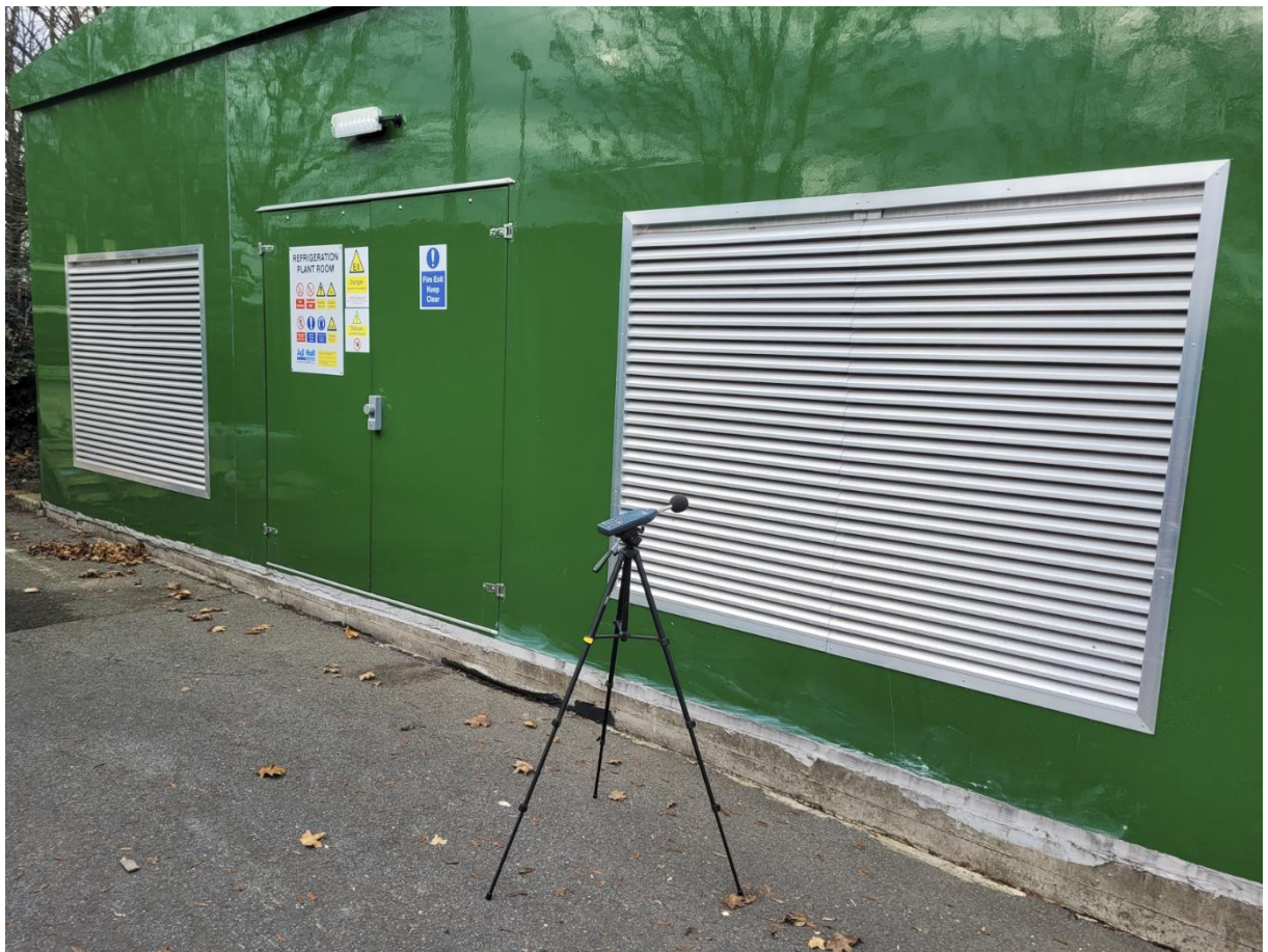
Figure D9: Ammonia Plant Room
