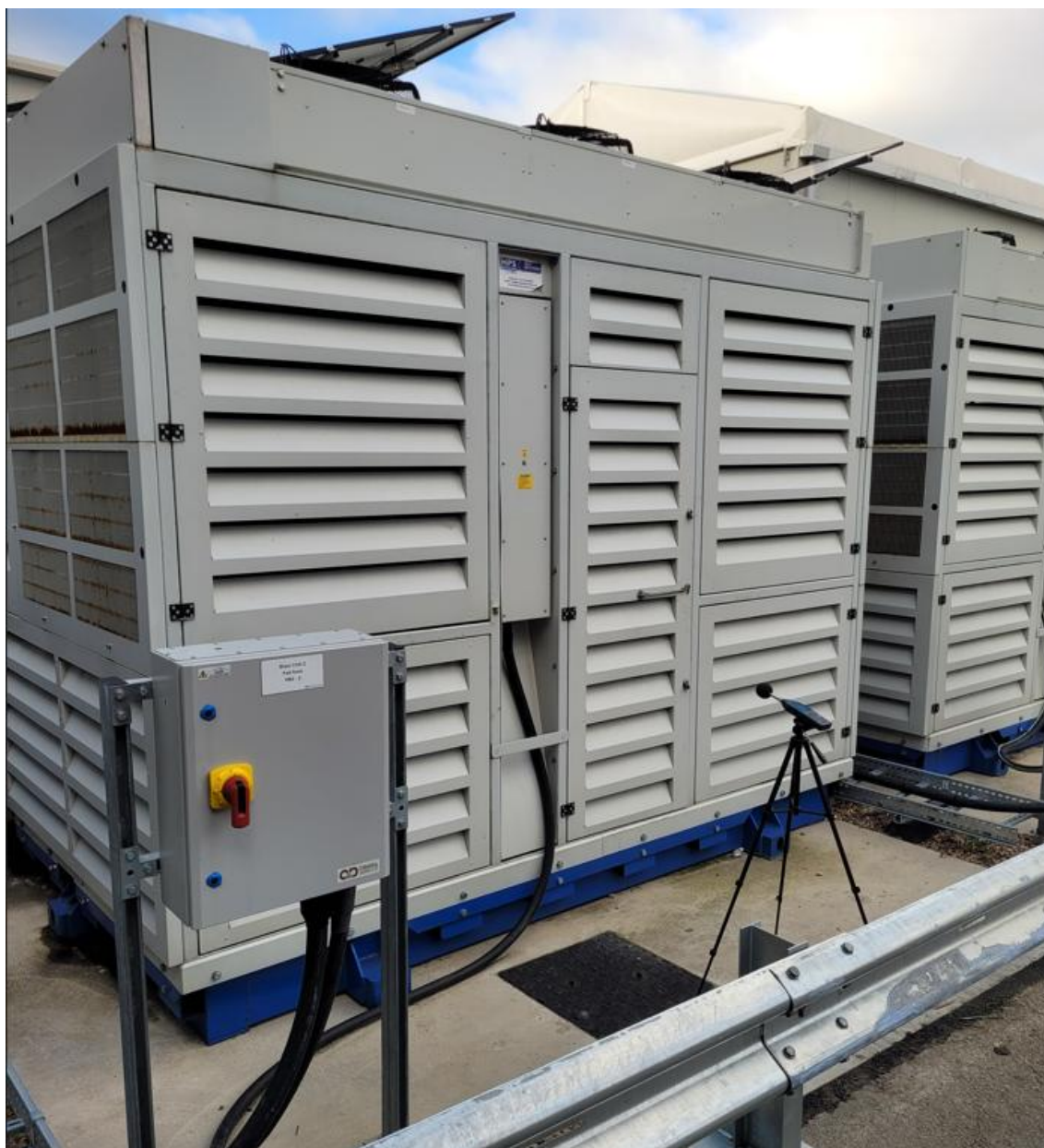
Figure D5: Blast Chiller
