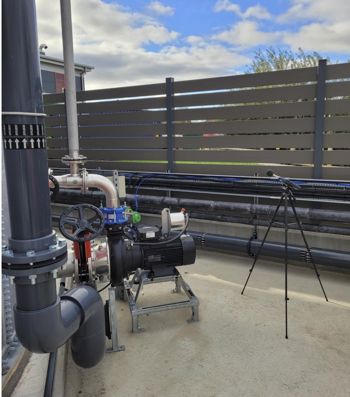
Figure D3: Effluent Pump
