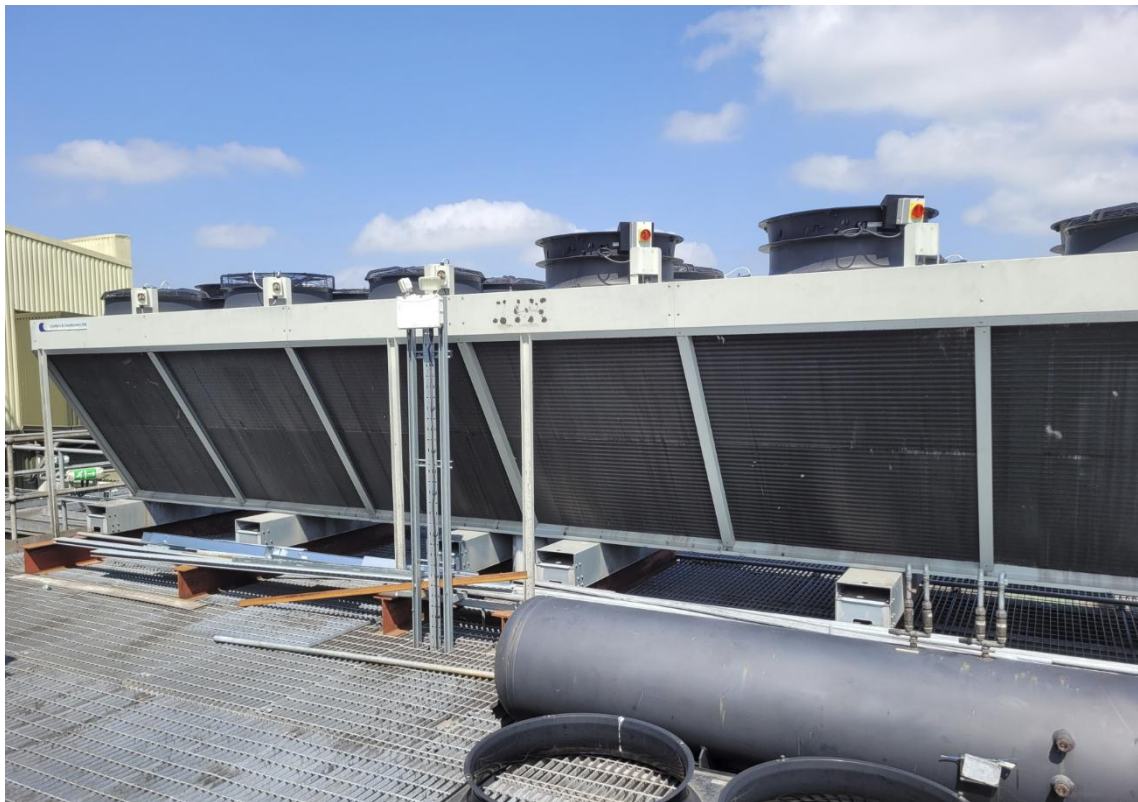
Figure D2: Cooler Condenser Units
