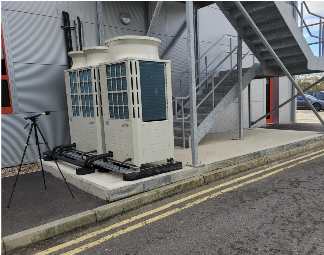
Figure D1: Chiller Units
