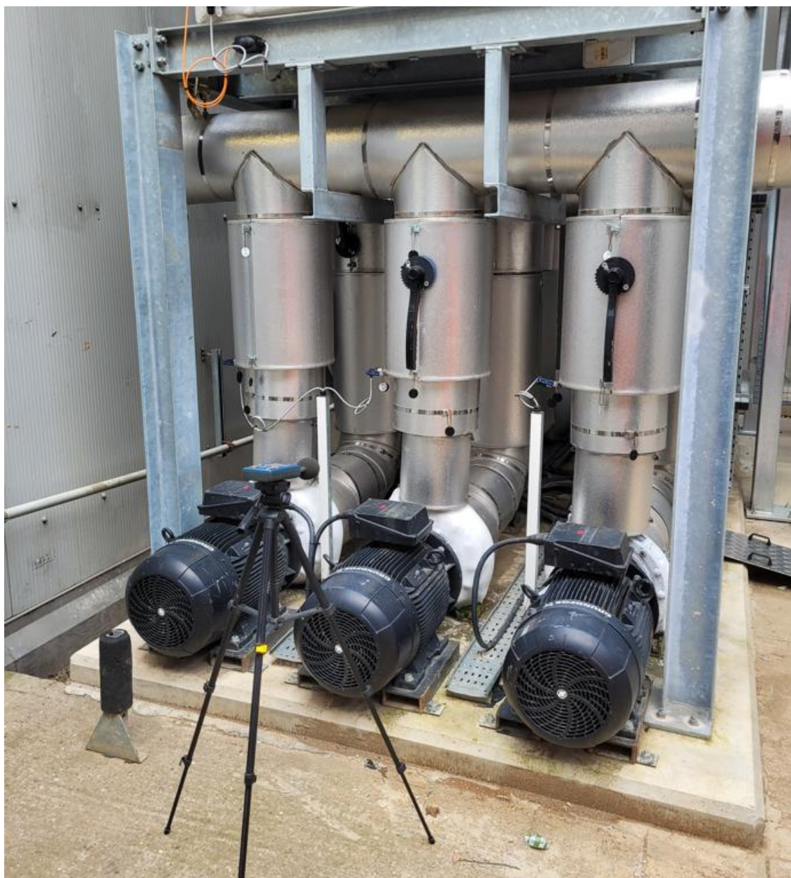
Figure D6: Glycol Pumps
