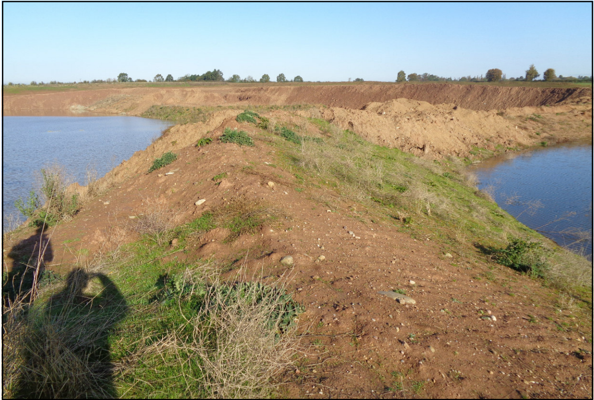
Photo 7. Differential head across dividing bund between flooded Phases 12/13 Excavation and restoration lake (RHS of photo).
