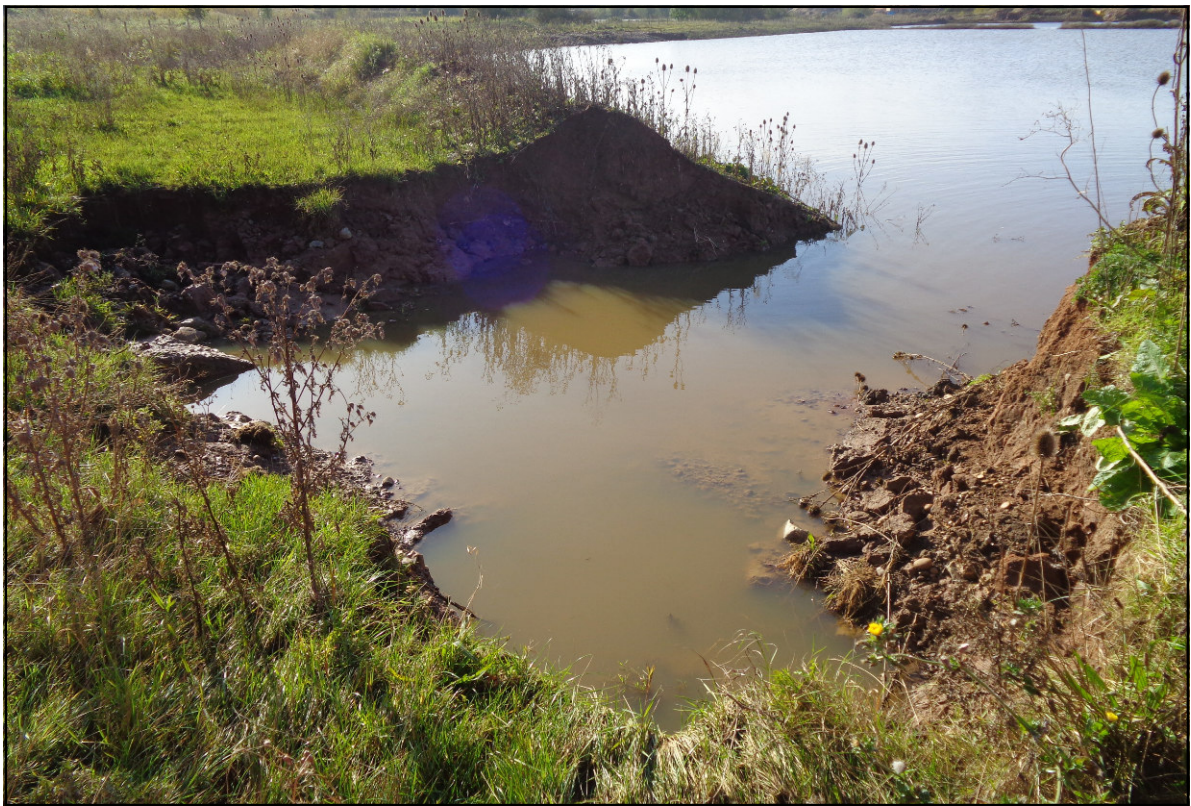
Photo 10. Surface erosion New Silt Lagoons.
