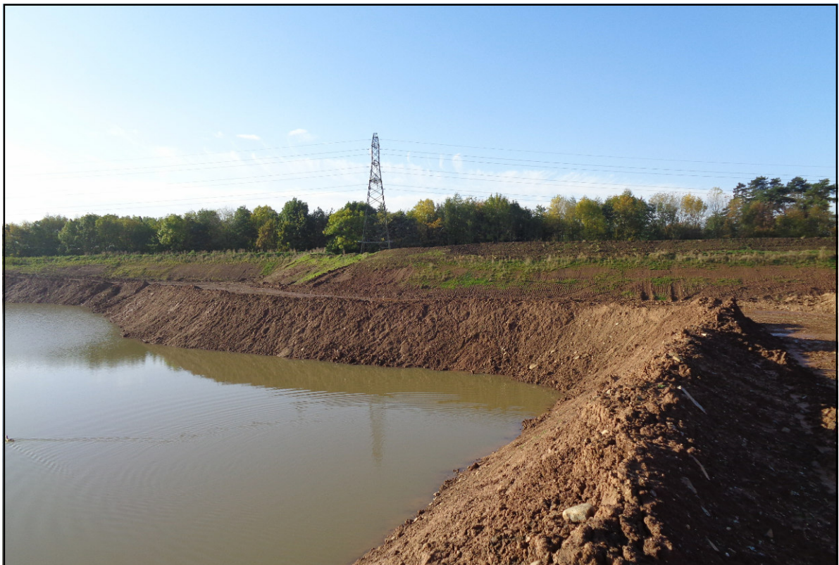
Photo 6. Electric pylon, seepage at toe of batter slope.
