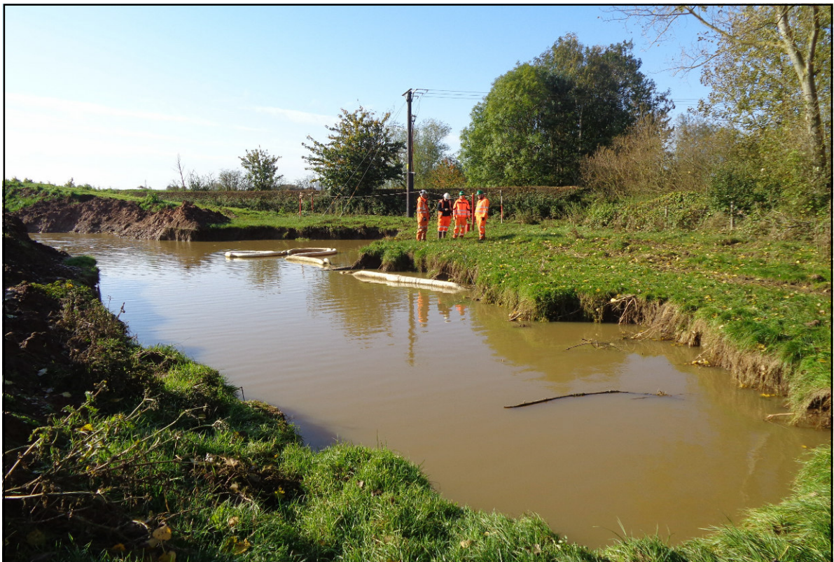
Photo 8. Flooded phase 2 excavation (area in front of personel) washed -out when brook flooded.
