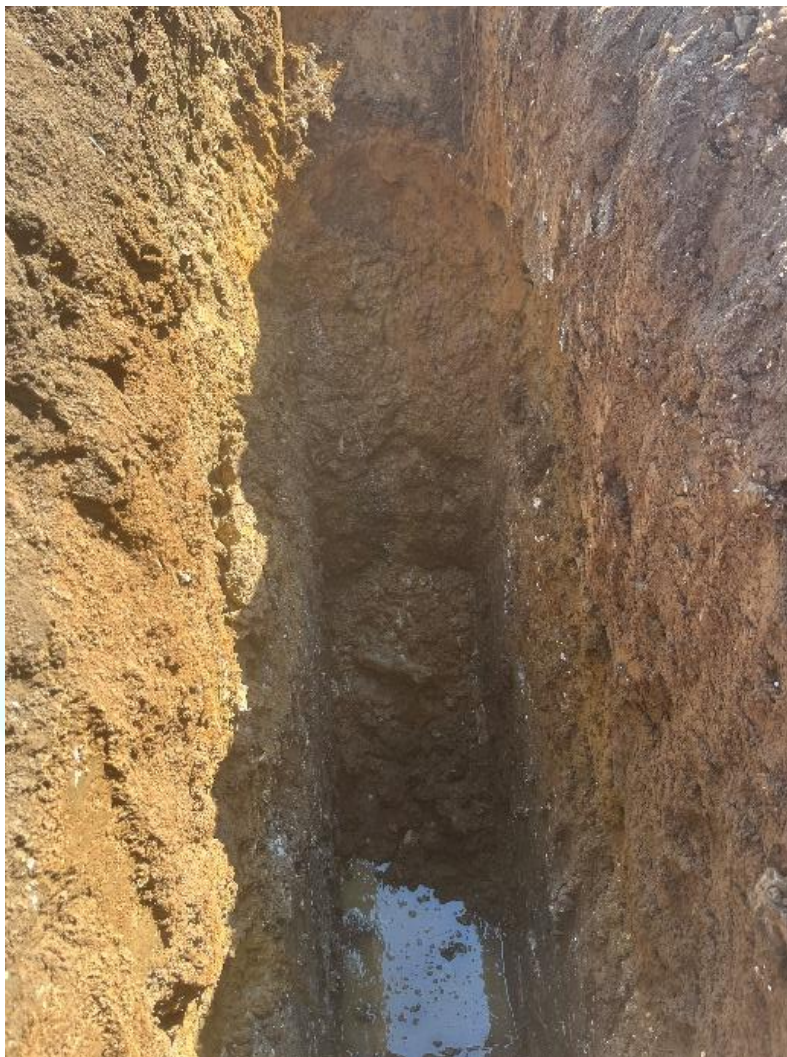
Photograph VI - Water seepage (TP105)
