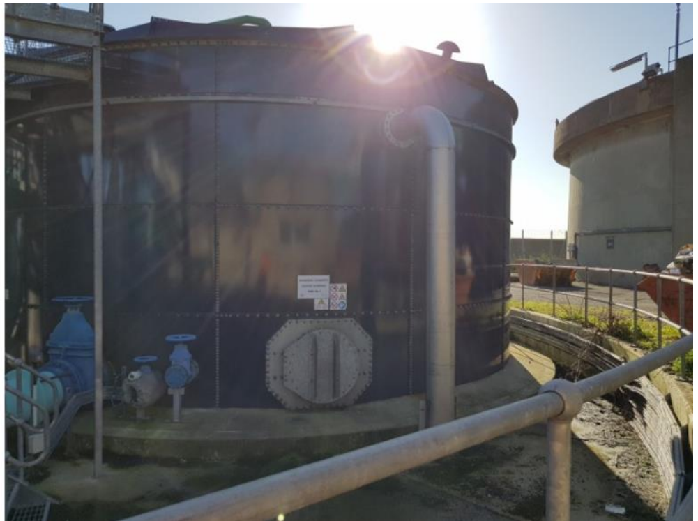
Photo of one of the Undigested Sludge Transfer Buffer Tanks, which receive screened Sludge prior to being transferred offsite.
