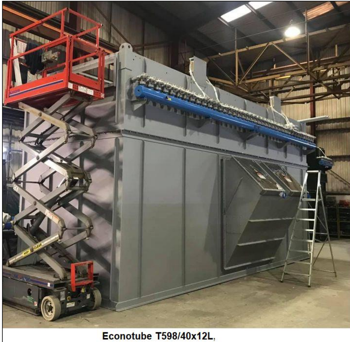
Figure 1-6 A Photograph of an Example of the Dust Extraction System
