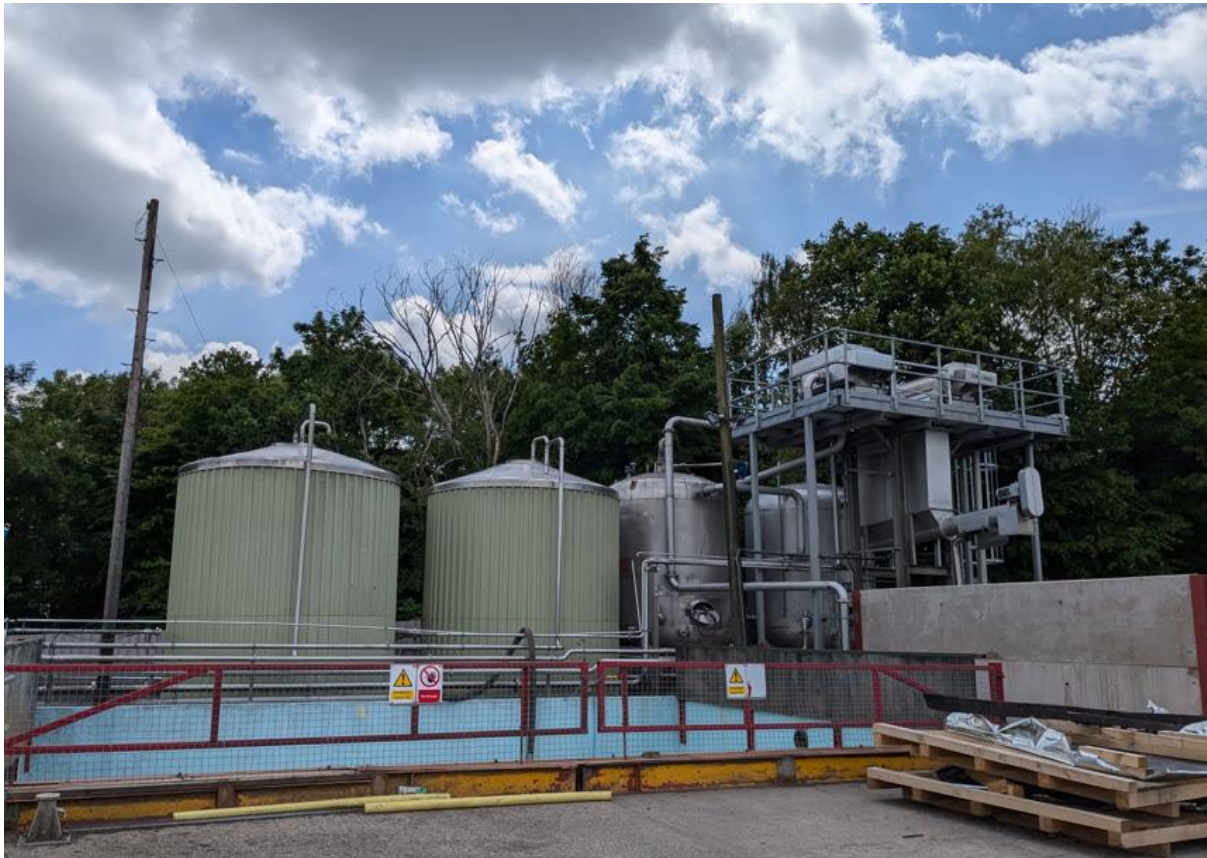
Photo 2: Water day tanks, recycled water tanks and filter press.
