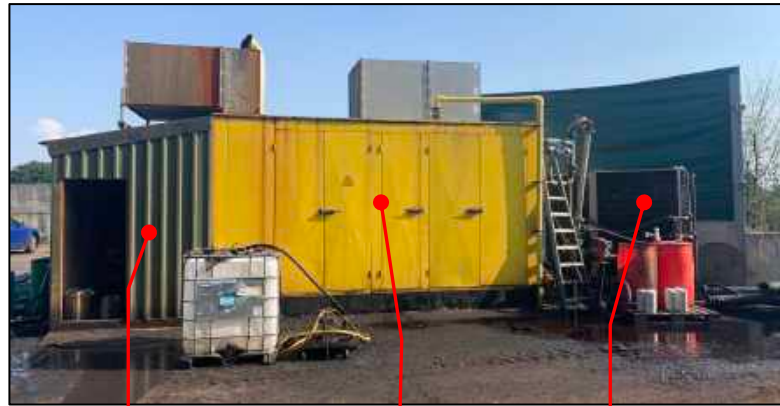
Control room CHP unit Cooling fans
