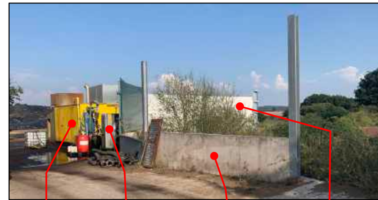
CHP unit Cooling fans 1.2m high concrete wall 3.6m high concrete wall
