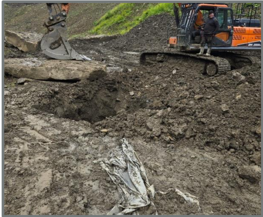
Plastic sheet found within the made ground in TP 4
