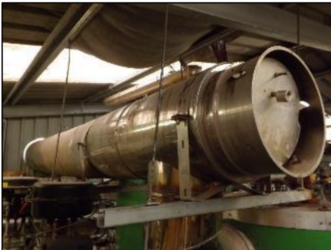
Figure 4.3: Horizontal Exhaust Pipe (internal)
