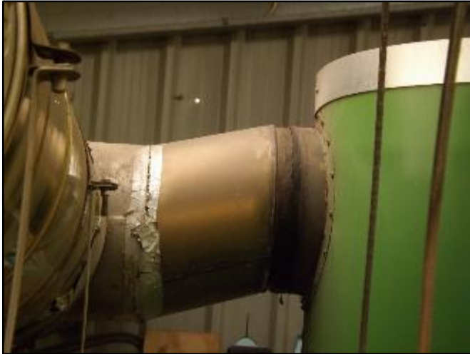
Figure 4.1: Boiler Exhaust (B-1)
