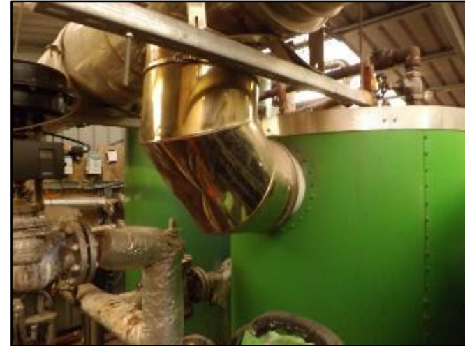
Figure 4.2: Boiler Exhaust (B-2)
