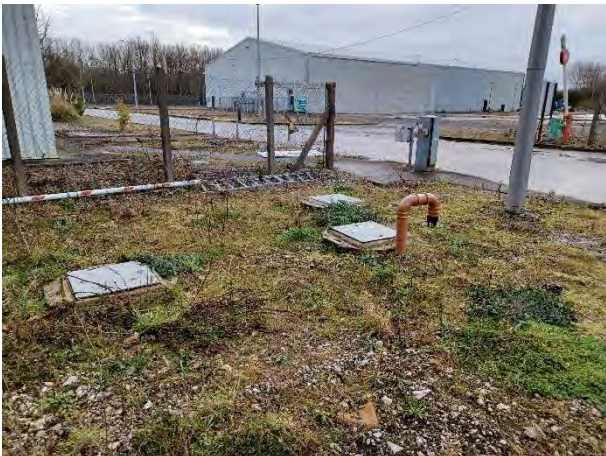
14.12.23 – Location of septic tank
