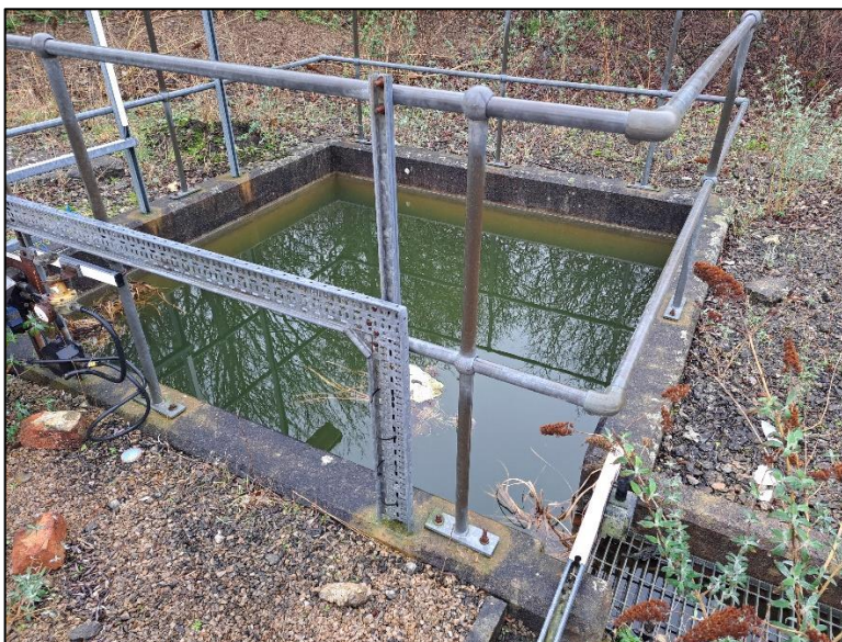
Photograph 8 showing standing water
