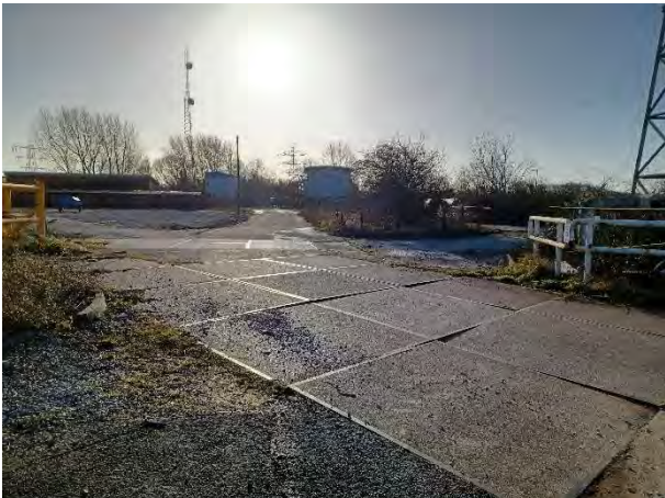
26.01.24 – Services access point in road
