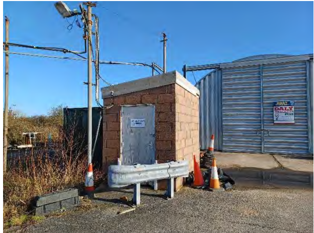
26.01.24 – Small substation powering Daley Cranes (off-site)
