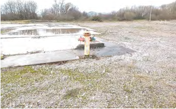
14.12.23 – Live fire hydrant located in the centre of site
