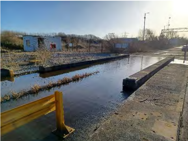
26.01.24 – View of bunded portion of road where tankers would off-load VCM
