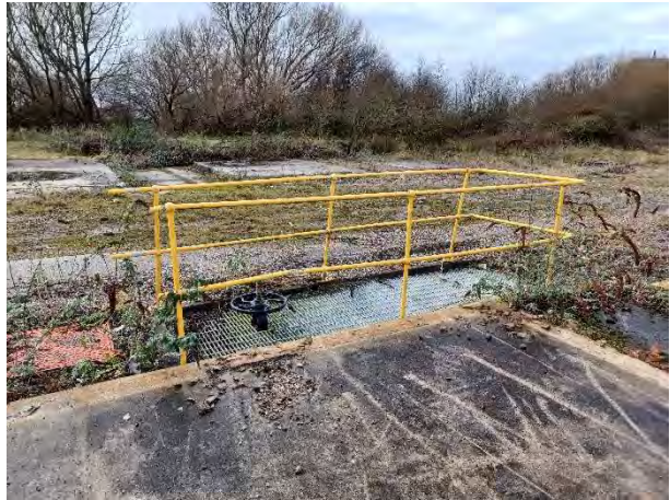
14.12.23 – Surface water drain access point near area of former mineralised water tanks
