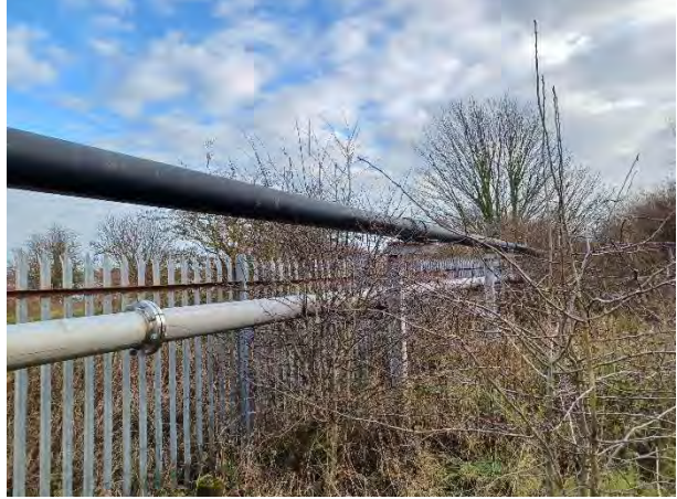
14.12.23 – View of treated water outfall pipes (off-site)
