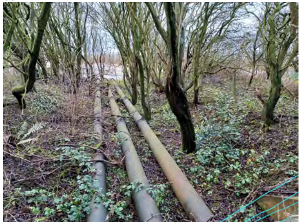
14.12.23 – View south of ethylbenzene pipes across habitat area in the north of the Site
