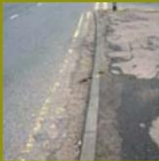
Grade D Heavily affected by detritus with significant accumulations
