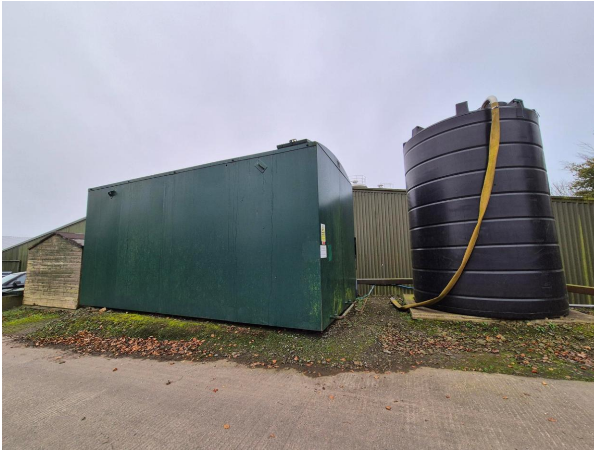
Photograph 11 –Bunded kerosene tank and water storage
