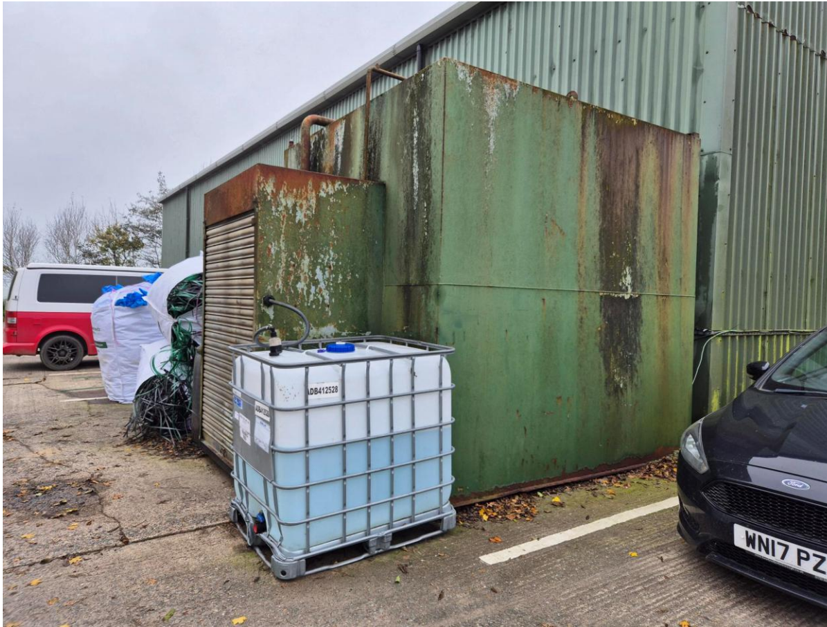
Photograph10– Bunded Diesel Tank (DERV Tank)
