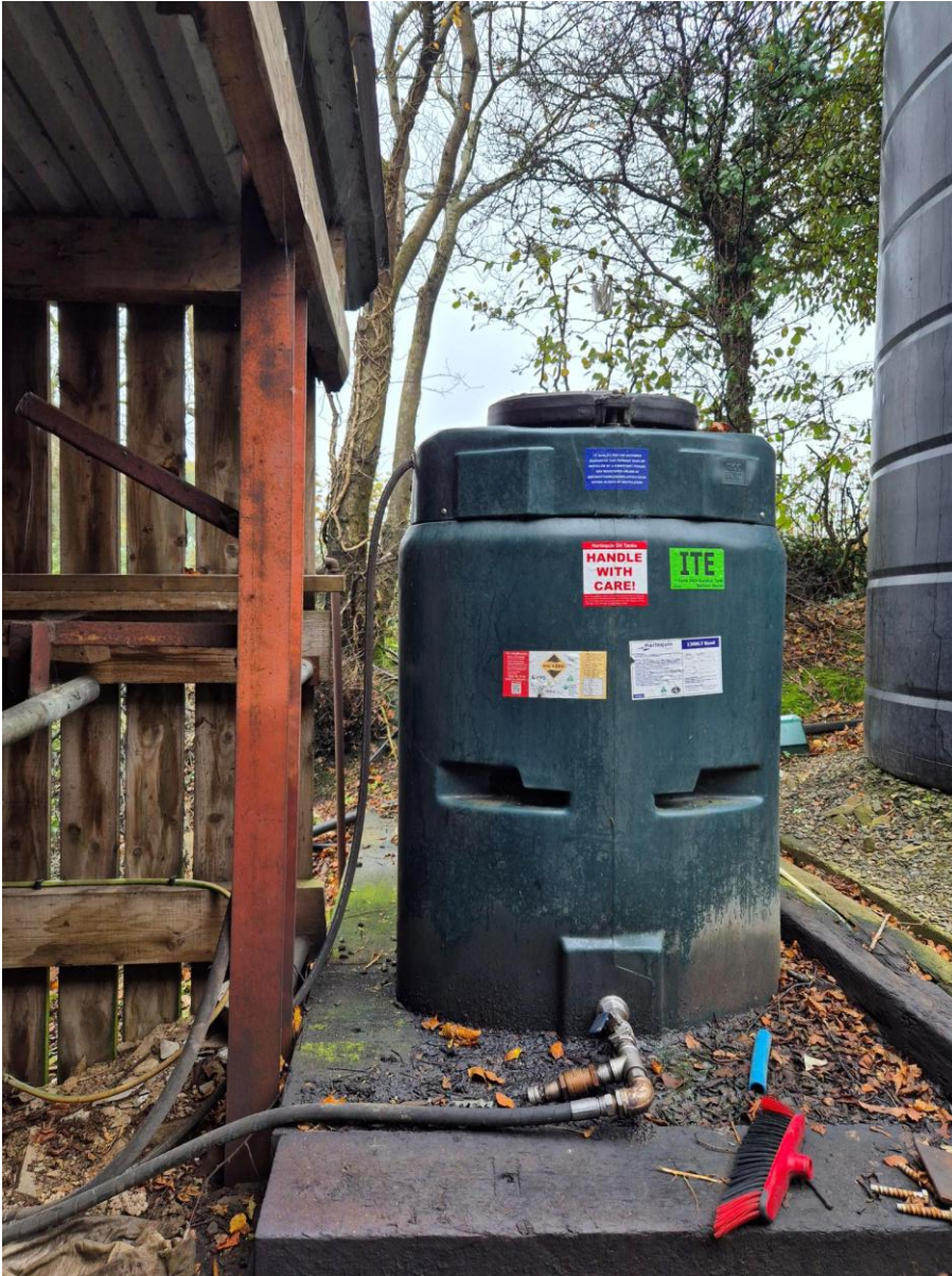
Photograph 12 –Bunded white diesel tank for generator
