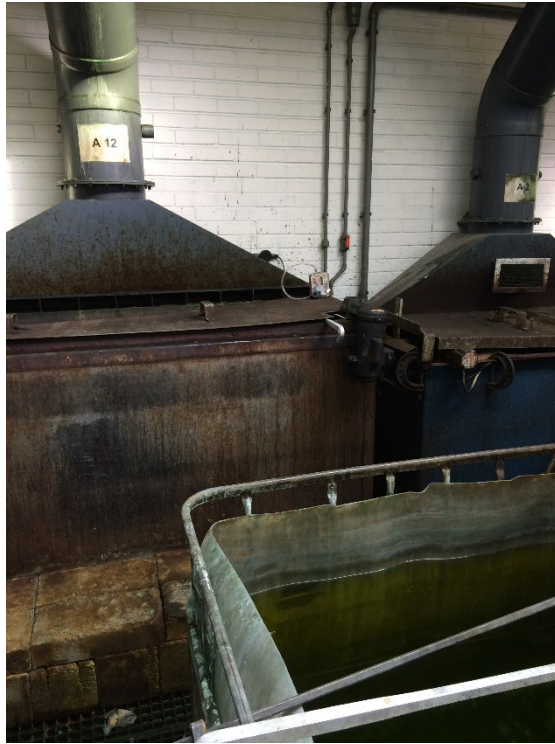
PHOTOGRAPH 1: A12 / A2 Tank Extraction Systems
