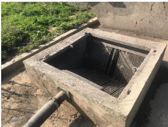
Plate 1. Grid inlet pipe and concrete surround.
