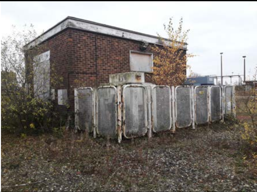
The electricity substation
