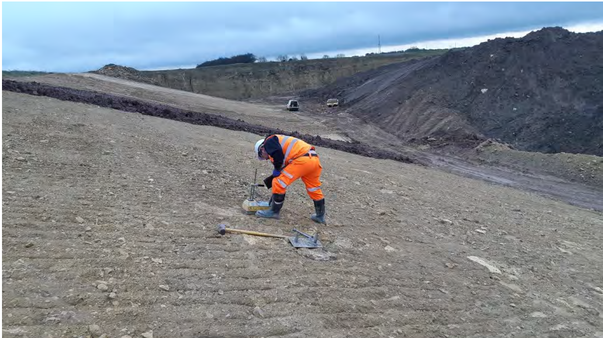
Testing on incomplete western area (eastern area to rear, beyond clay bund)
