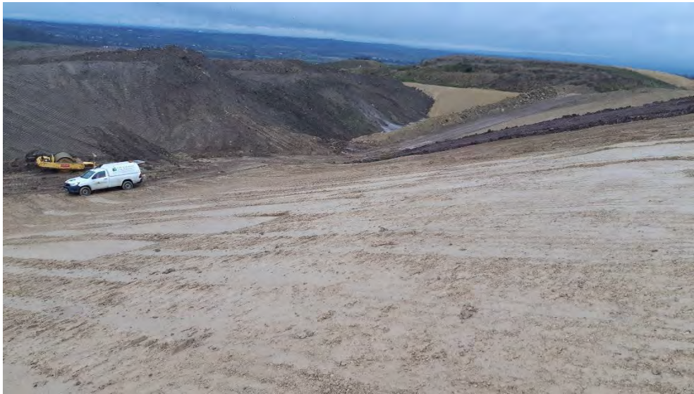
Compaction on east part of Phase 1 north batter slope. Note clay dividing bund separating east and west areas to upper right of photograph
