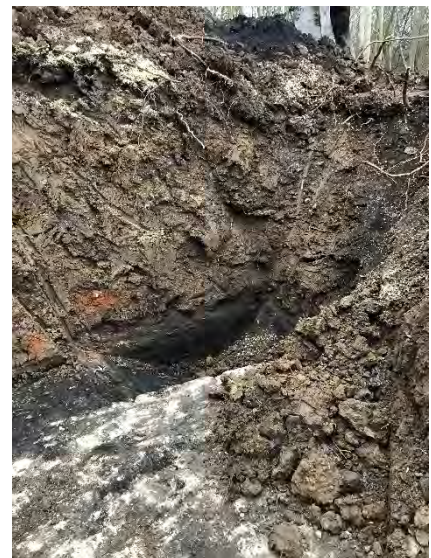
Photo No. 5 - 433550-003 North Eastern Edge of Concrete
