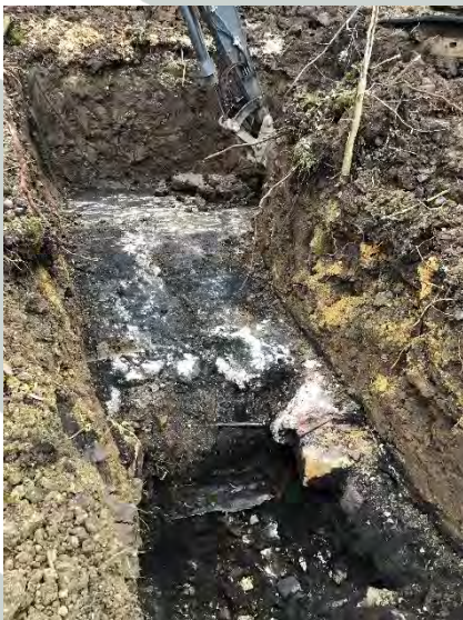
Photo No. 3 - 433550-003 Southern Edge of Concrete
