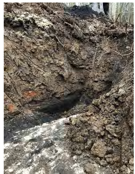
Photo No. 5 - 433550-003 North Eastern Edge of Concrete
