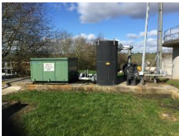
Figure 6: Moderator/ Peacemaker Odour Control Unit on sludge transfer well
